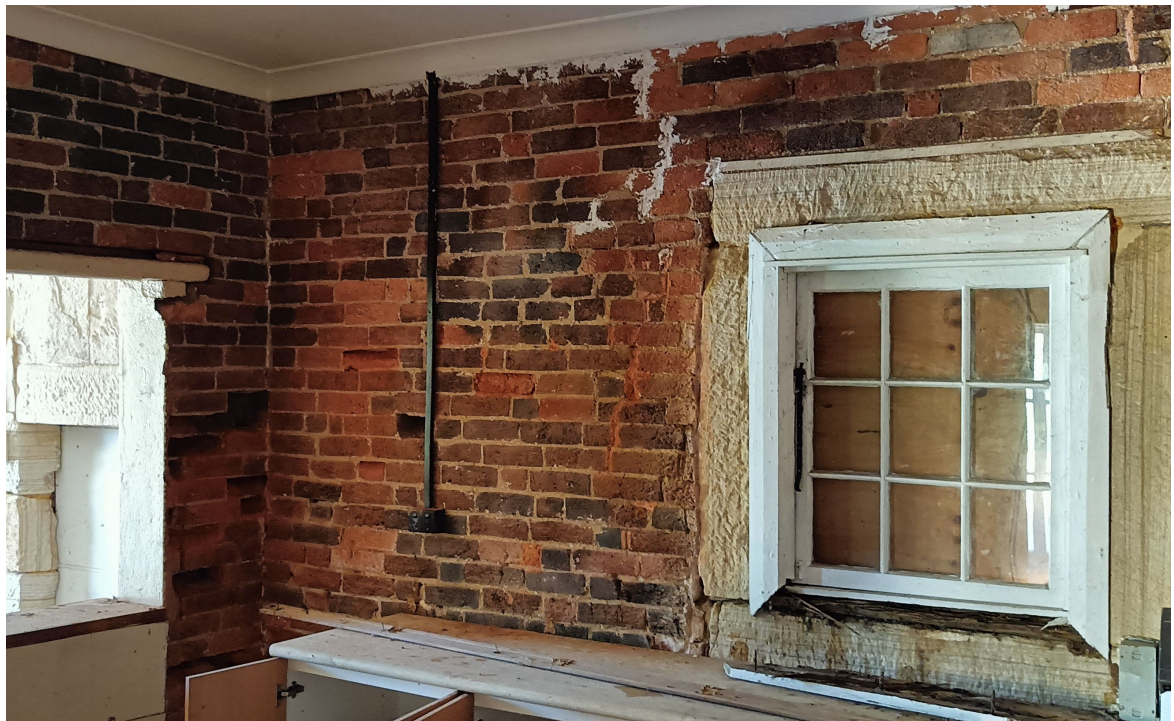
Plate 47. North-east corner of the brick structure. Various materials can be seen to have patched damaged areas (Source: Archive Heritage)
