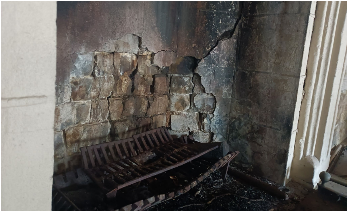
Plate 41. Detail of the fire bricks used beneath the cracked render (Source: Archive Heritage)
