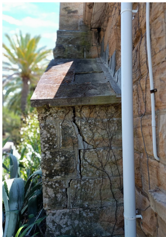
Plate 21. Cracking on the chimney seen from the south (Source: Archive Heritage)
