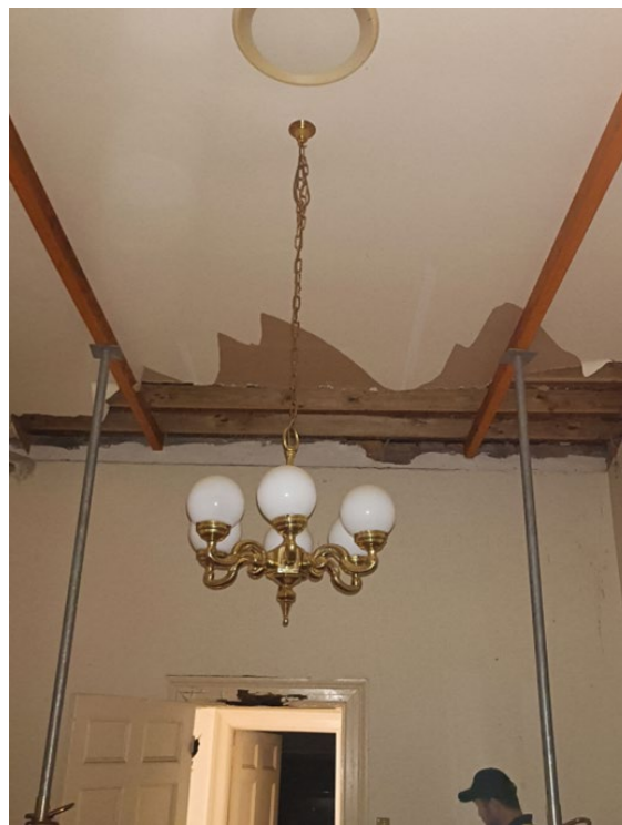
Plate 25. 20 th View north of the Dining Room showing ceiling damage (Source: Archive Heritage)
