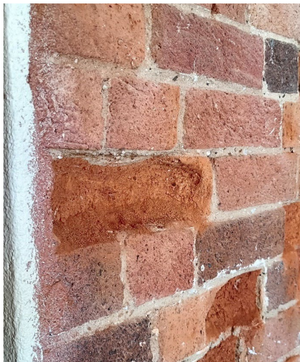
Plate 49. Detail of mortar and spalling brickwork (Source: Archive Heritage)
