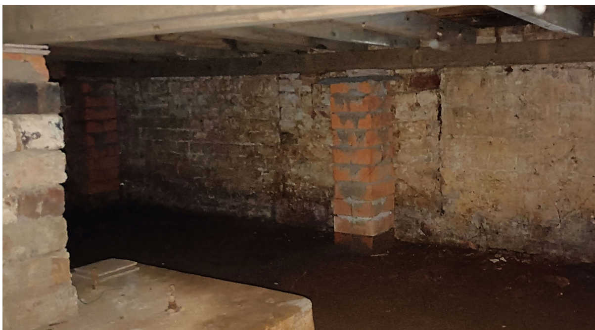
Plate 54. Possible original, in-filled entry to the Phase 1 brick building's cellar, seen behind the modern brick floor support pillar (Source: Archive Heritage)
