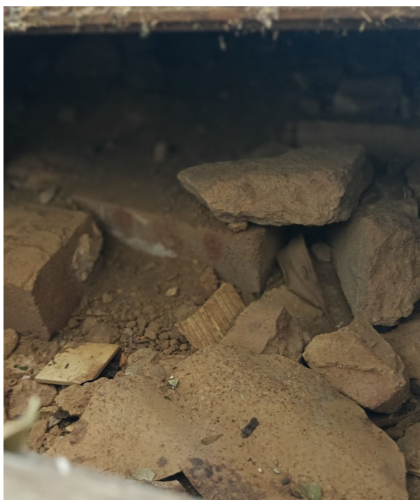
Plate 12. Disused timber support pad materials from previous phases of decking (Source: Archive Heritage)
