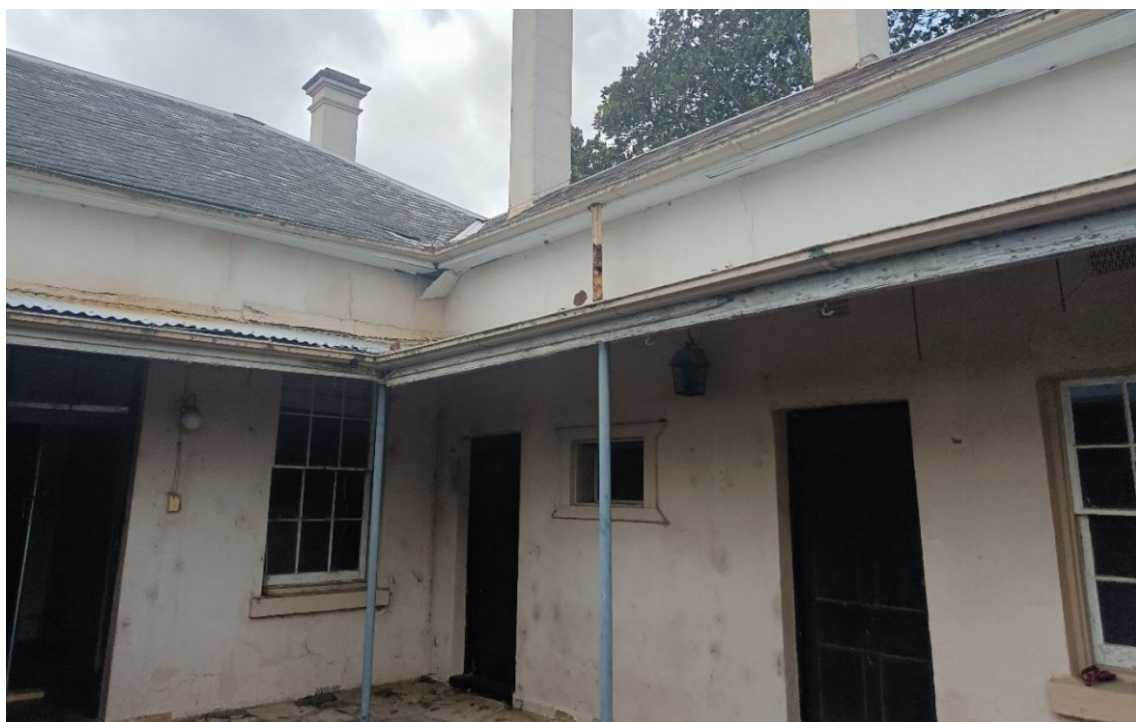
Plate 28. View south-east of the start of the South Wing. Failed roof plumbing is seen at junction (Source: Archive Heritage)
