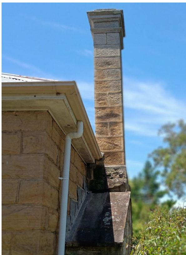
Plate 20. Tilted chimney seen from the north (Source: Archive Heritage)
