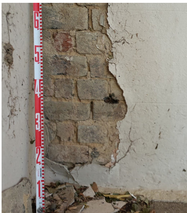
Plate 14. Fallen render and exposed masonry (Source: Archive Heritage)
