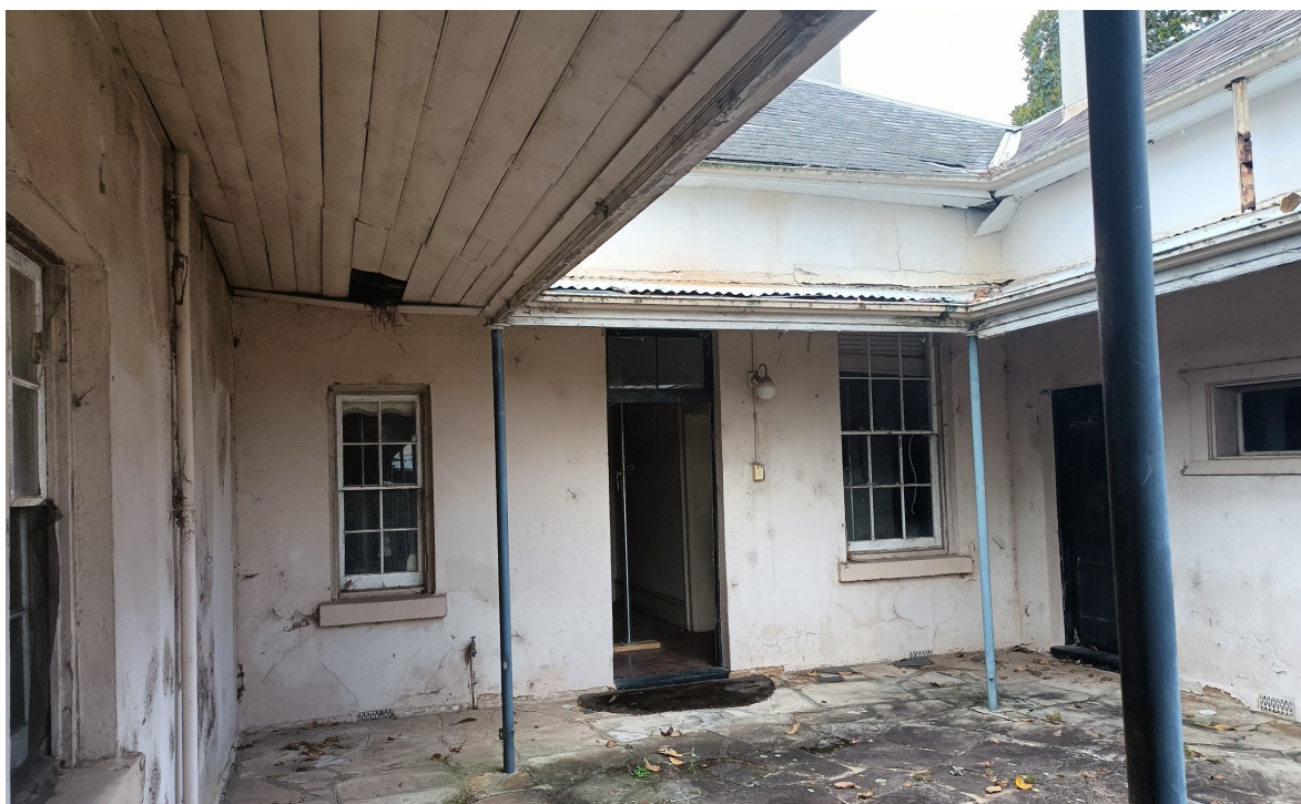
Plate 23. Courtyard doorway and altered window reveals at the back of the Main House. Failing flashing and eaves are visible (Source: Archive Heritage)
