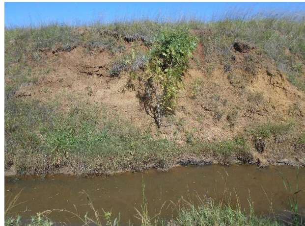
Plate 14: General photo of the Subject Area showing soil erosion along bank of Foot Onslow Creek.
