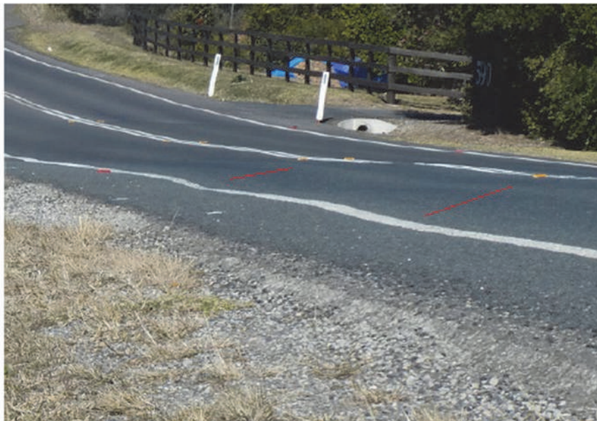
Fig. 6.3 Compression bumps in Menangle Road (Source: Network Solutions)
