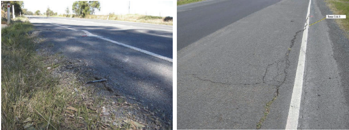
Fig. 6.4 Bump in slip lane along Appin Road above West Cliff Longwall 32 (Source: Colin Dove)
