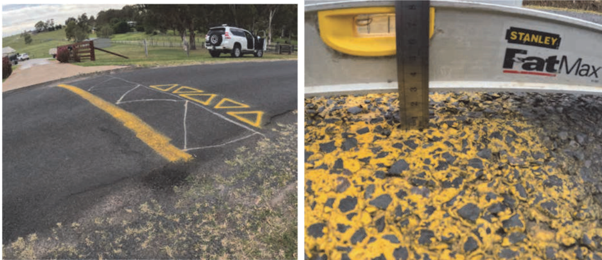
Fig. 6.2 Bumps and dip along Carrolls Road above Appin LW710B (Source: Inglis, 10 Oct 2024)
