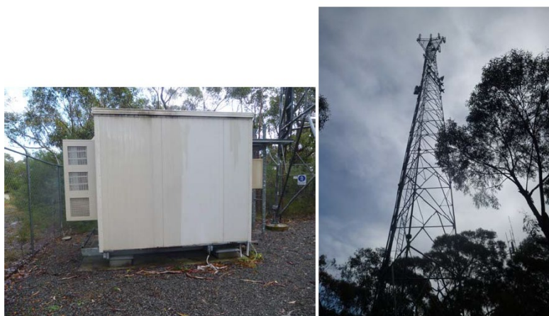
Plates 3 & 4 – Telecommunications Tower 2 and Compound (Source: MSEC, 2016)
