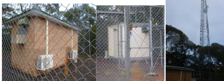
Plates 1 & 2 – Telecommunications Tower 1 and Compound (Source: MSEC, 2016)
