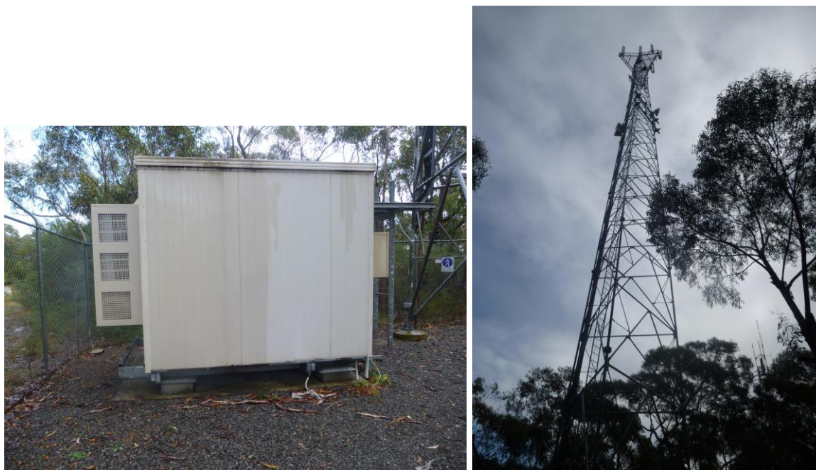
Figure 2 Axicom Telecommunications Tower 2 and Compound
