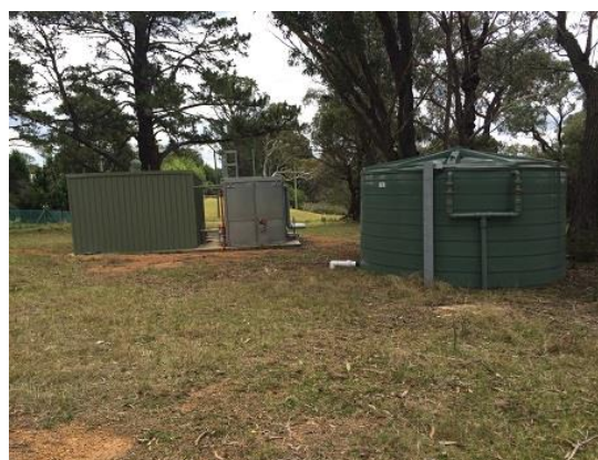
Figure 9 Water Storage Tanks Refs. B17t01 (poly tank) and B18t01 (steel tank)
