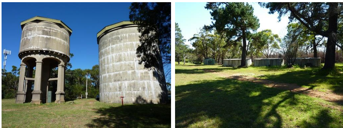
Figure 8 Water Storage Tanks Refs. B14t01 and B14t02 (left side) and Refs. B16t01 to B16t03 (right side)
