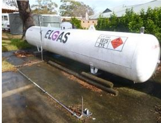
Figure 10 Gas Storage Tank B01t03
