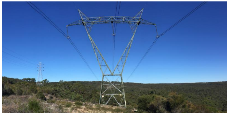
Figure 1 Photograph of a 330 kV Transmission Tower
