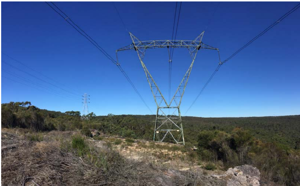
Figure 1 Photograph of a 330 kV Transmission Tower
