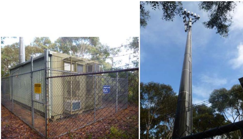
Plates 1 & 2 – Telecommunications Tower and Compound (Source: MSEC, 2016)
