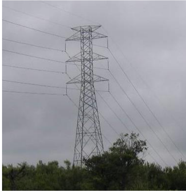
Figure 1 132 kV Transmission Tower
