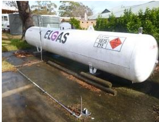
Figure 10 Gas Storage Tank B01t03
