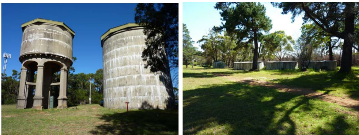
Plates 15 & 16 – Large Water Storage Tanks (Source: MSEC, 2016)
