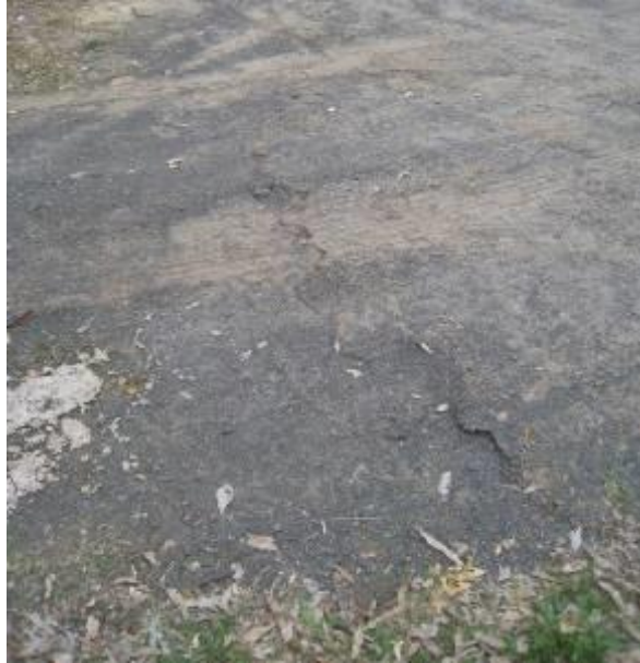
Fig. 4.14 Surface Compression Buckling Observed in a Pavement
