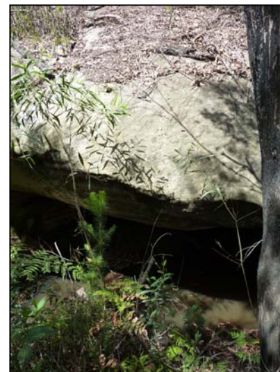
TB100-6 Overhang on southern bank
