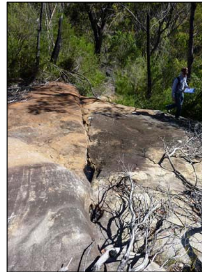
TB069-6 Joint with water
