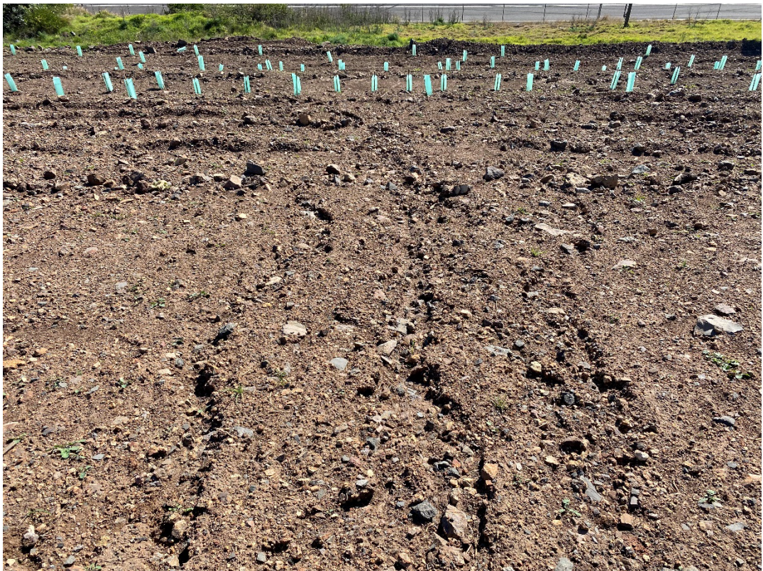
Photo 12: Minor rill erosion forming in overburden area on northern side of site. Note that a Sediment Dam and additional erosion control is recommended for this area.
