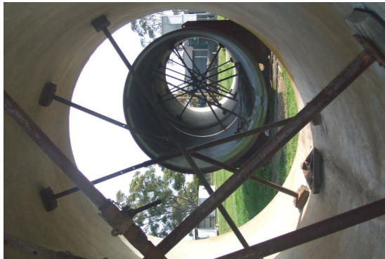
Defunct water carrier pipes with structural re-enforcement
