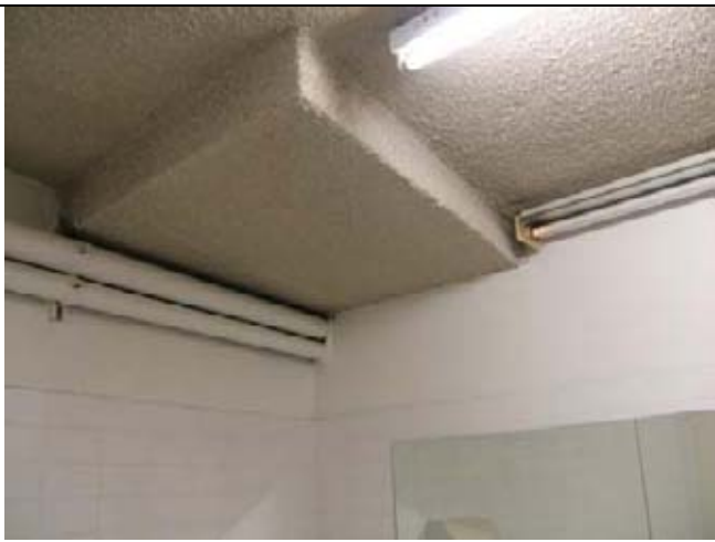
Plate 3: Sprayed fibro material in the toilet facility. The same material was noticed in several areas of the Travelex premises
