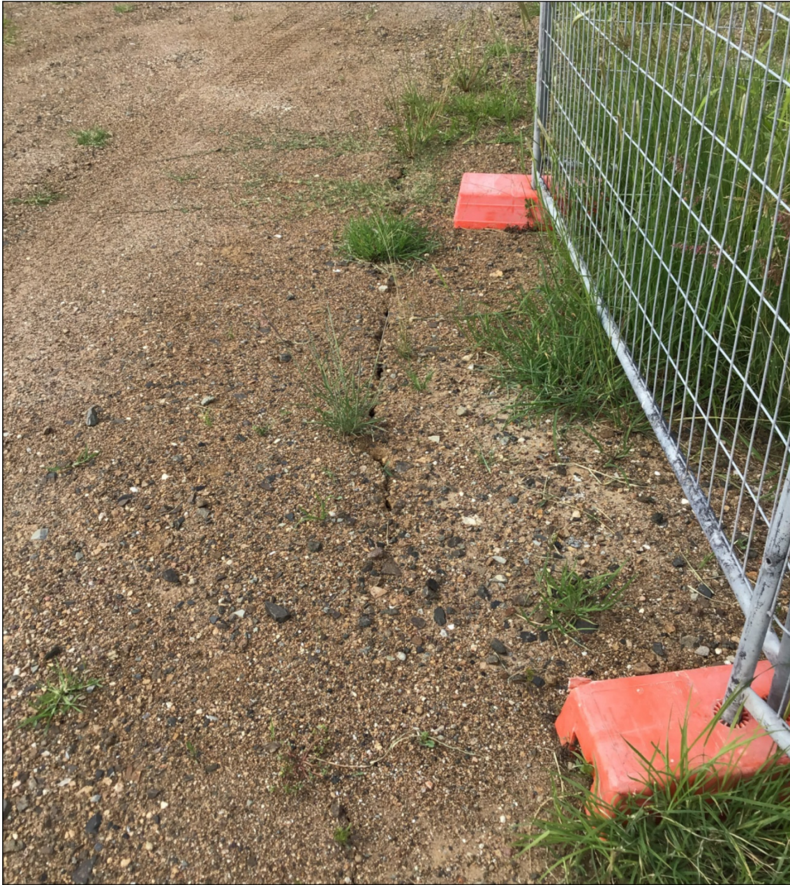
Figure 2: Surface crack at gas drainage pad on causeway.
