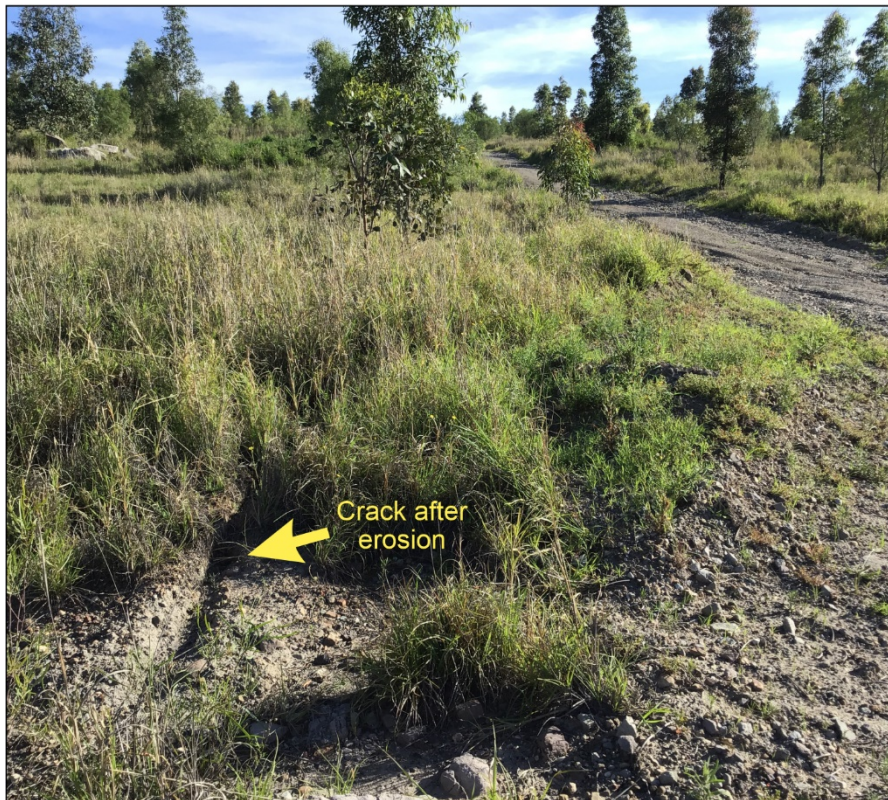
b) Surface crack on 16 November 2020.
