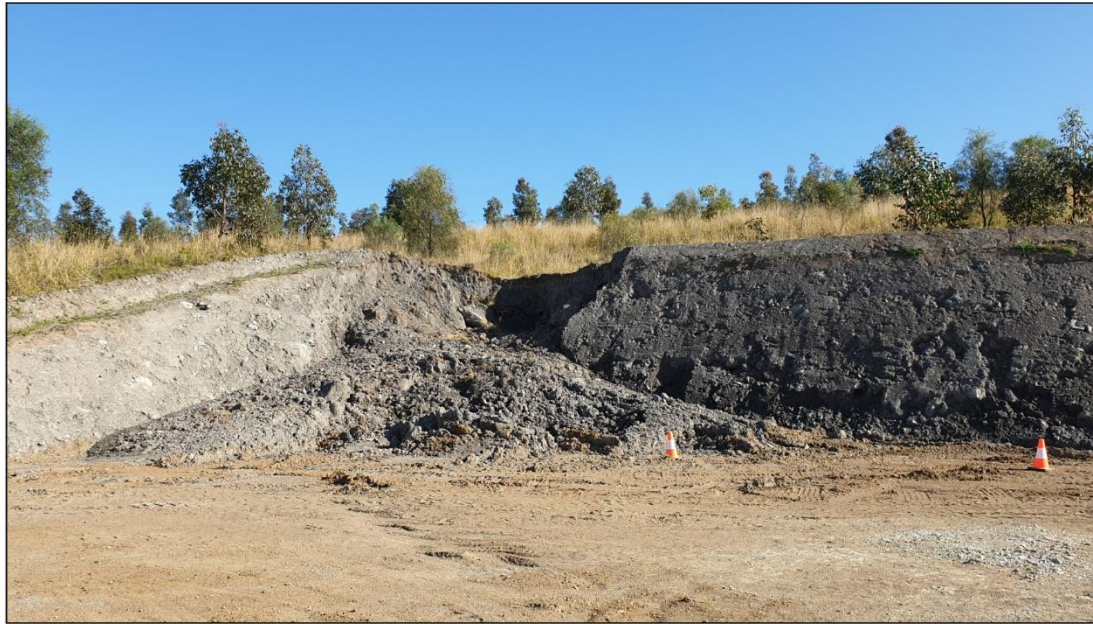
a) Erosion at top bank of Gas Drainage Pad.
