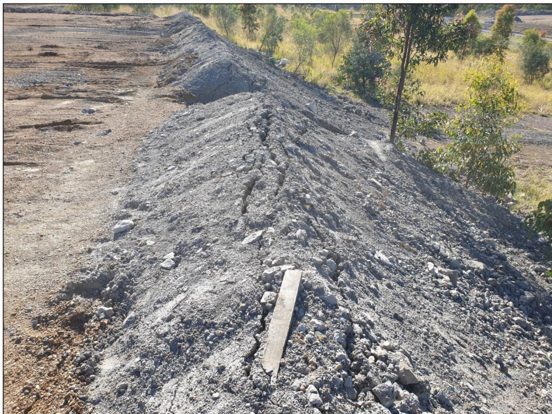
b) Settlement or slumping of bunding and bottom batter slope of Gas Drainage Pad.
