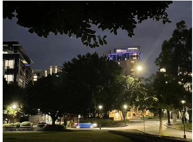
View from Wharf Street: This view has been designed specifically using energy efficient, dimmable, adjustable fixtures with glare guards and louvers preventing unwanted glare and spill light.
