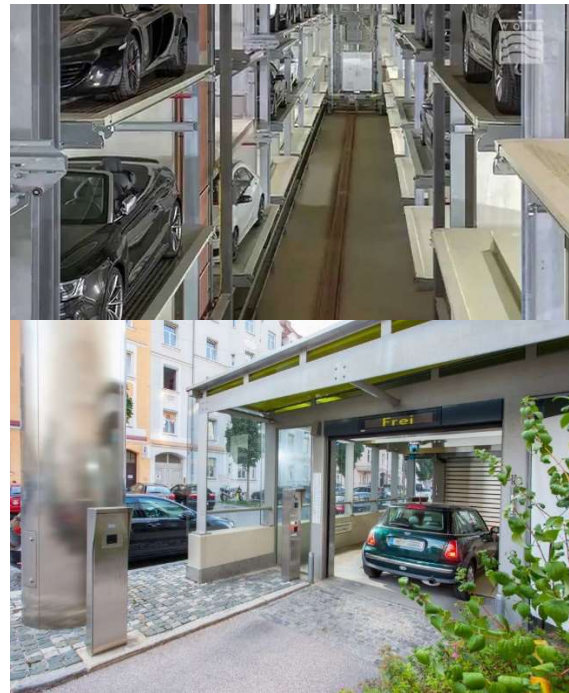
Figure 3.8: Multi-parker Stacker Car Park System
