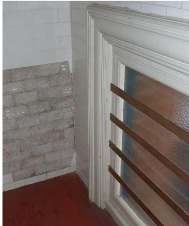
Picture 63 ĩ Window on landing of secondary northern stair. Note need for tile repair.
