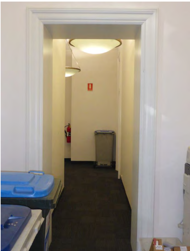
Picture 85 i Typical opening in corridor with architrave but no door leaf.
