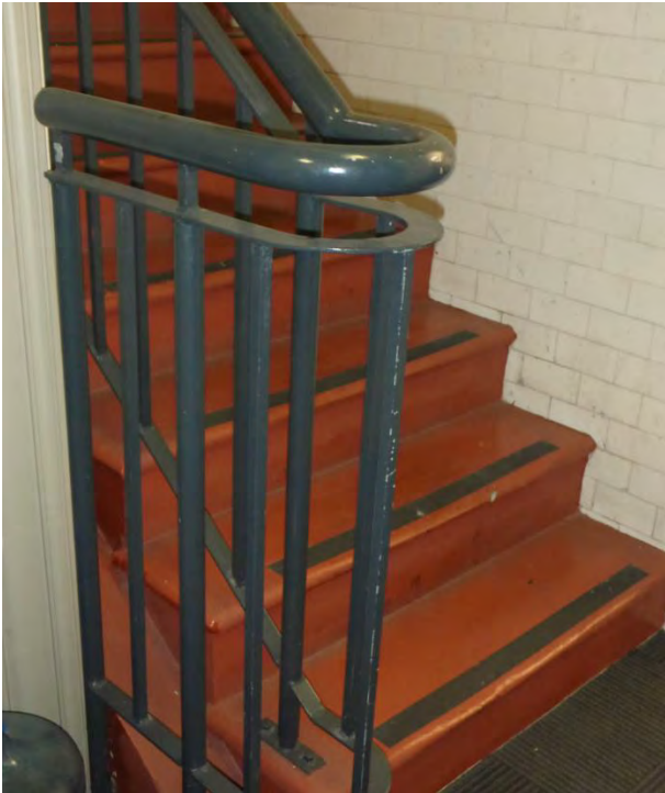
Picture 62 ĩ Secondary (northern) staircase. Note addition of higher circular handrail to comply with NCC.
