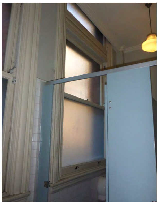
Picture 52 i Window in the ground floor bathroom. Note false ceiling drops below top of window head.
