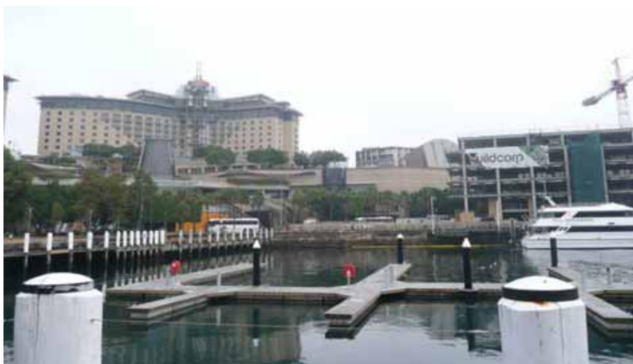
PHOTOGRAPH LOOKING ACROSS PYRMONT BAY TOWARDS THE NORTHERN TOWER OF THE CASINO AND THE NEW DEVELOPMENT UNDER CONSTRUCTION ON PIRRAMA ROAD AND THE SOUTHERN END OF DARLING ISLAND
