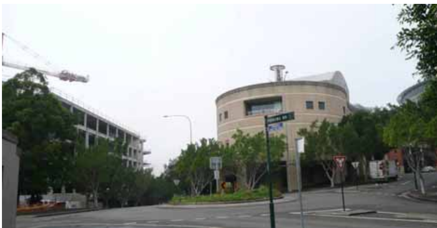
PHOTOGRAPH LOOKING AT THE INTERSECTION OF JONES BAY ROAD WITH PIRRAMA ROAD WITH THE CURVED END OF THE EXISTING CASINO VISIBLE AND THE NEW 5 STOREY DEVELOPMENT UNDER CONSTRUCTION ALONG PIRRAMA ROAD
