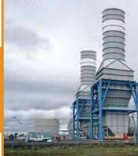
Gas-fired power plant
