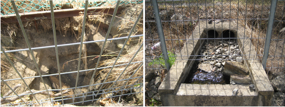
Figure 5.2 Ageing drainage systems found at the EASTERN end of the project site.
