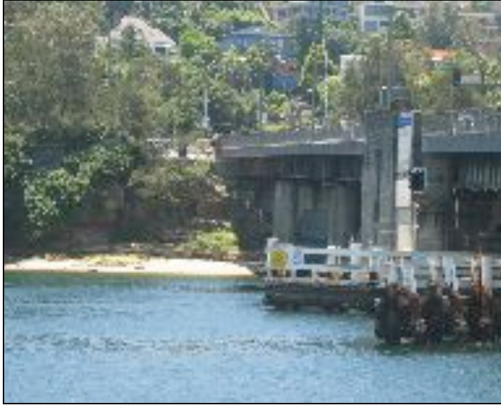
Figure 7: Five concrete stub pillars at the northern abutment of the first Bridge.
