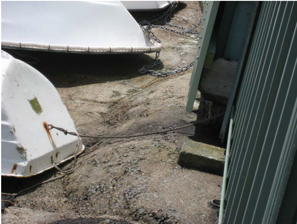
PHOTO NINE: Oil staining outside of waste storage compound heading towards Lake Macquarie (AEC 4).
