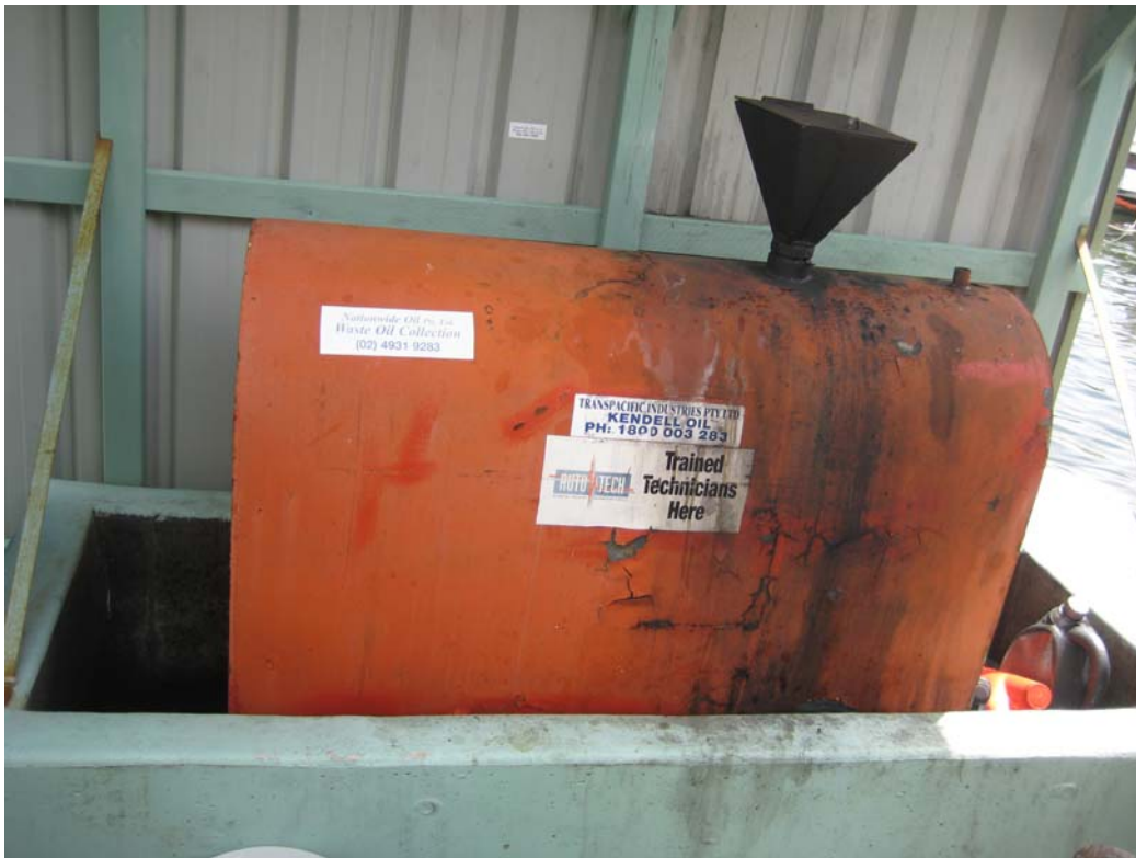
PHOTO EIGHT: Waste motor oil AST in waste storage compound (AEC 4).
