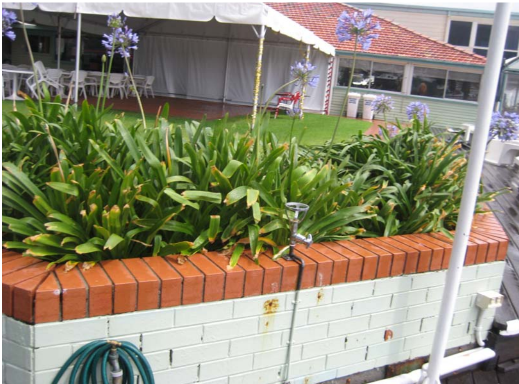
PHOTO TWO: The garden bed and undercover area on western side of yacht club building.
