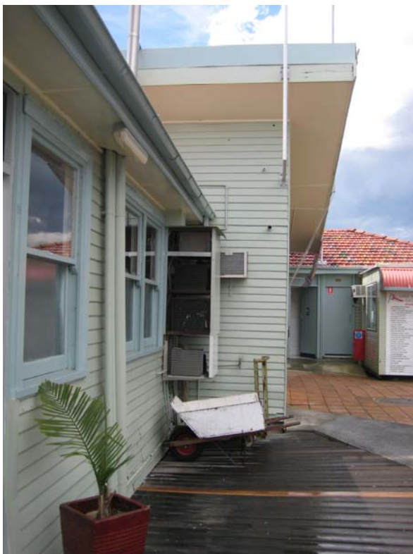
PHOTO SIX: Entrance to yacht club building. Potential asbestos containing material in eaves lining (AEC 3)
