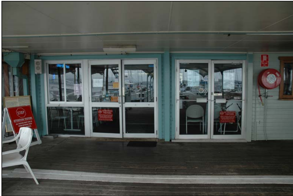
Photo 7 Inclusion of unsympathetic fabric - rear of building.
