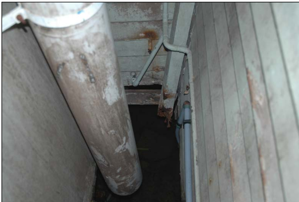
Photo 10 An example of support structures subject to rot.
