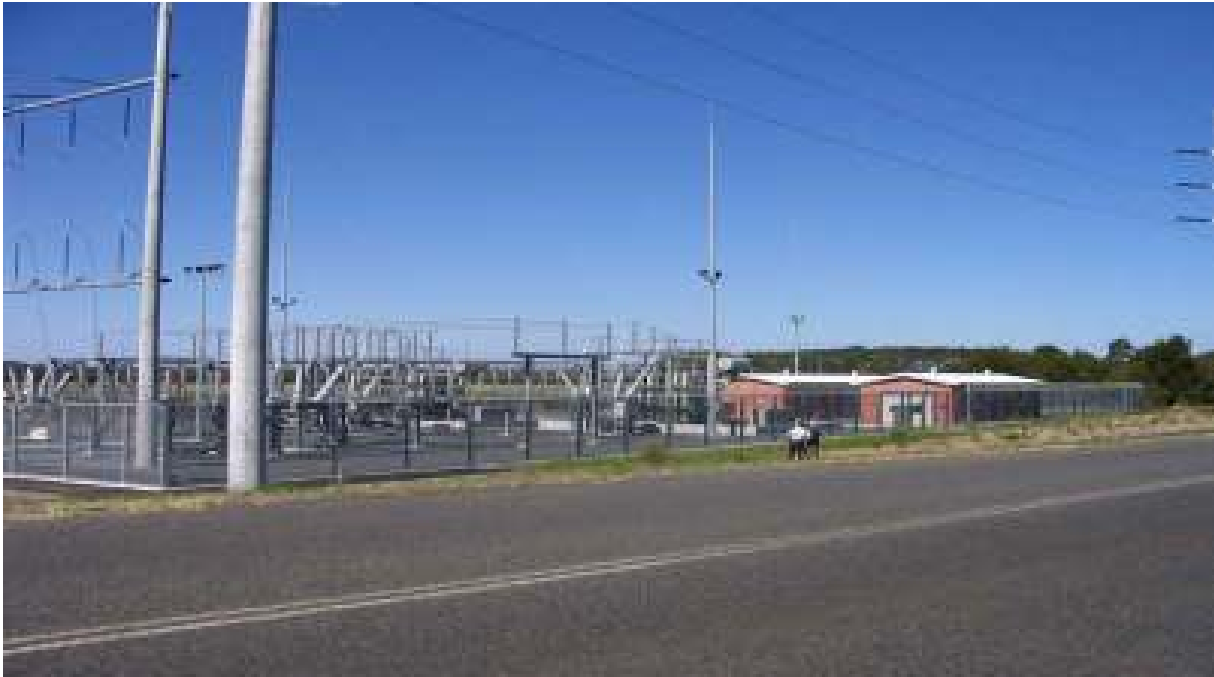
Figure 12: Example of Substation Similar to that Proposed for Suffolk Park
