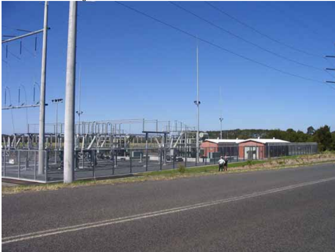
Figure 3-7: Similar substation design at Lennox Head
