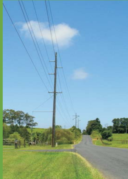
Existing 66kV infrastructure near Ewingsdale
