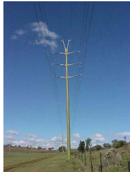
Example of a dual circuit powerline
