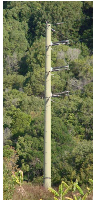
Example of 132kV powerline
