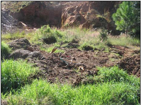
Plate 10. Fill material with general rubbish
