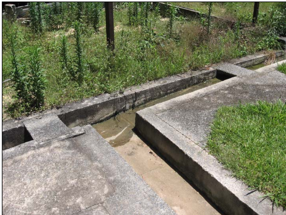
Photo 2: Stormwater drainage system.
