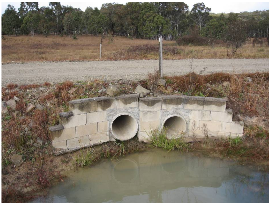
Figure 2-4 Canyonleigh Road showing faulty pipe culverts
