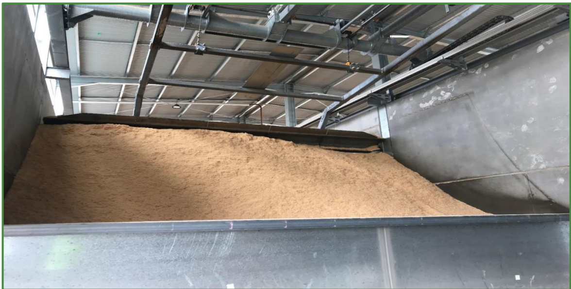
Figure 2-1: Sawdust used in Biomass Boiler
