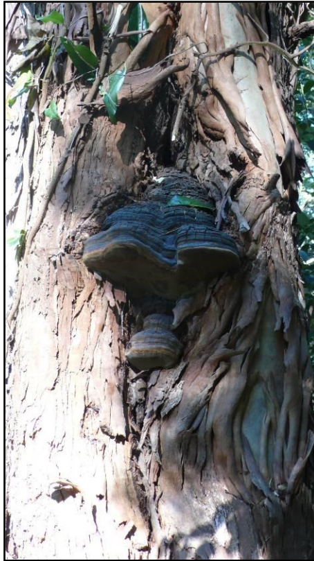
Photo A: Fungal bracket creating a structural defect in base of T323. Tree recommended for removal despite being clear of proposed construction.
