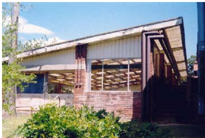
Figure 60: The enclosure around the swimming pool has deteriorated and it is in fair condition only. Although an important adjunct to the treatment of children, it is not in sympathy with the pool of nearby “Rippon Grange” (Rod Howard Heritage Conservation Pty Ltd, October 2000).
