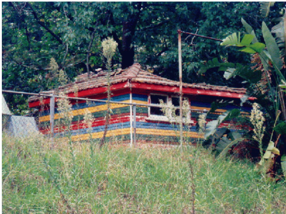
Figure 73: Killara Cottage. Photograph taken in March 2006 showing serious deterioration (Rod Howard & Associates).
