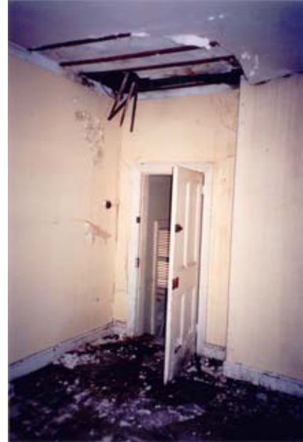
Figure 142: Damaged ceiling fabric, Room F19 (Rod Howard & Associates, 2006).
