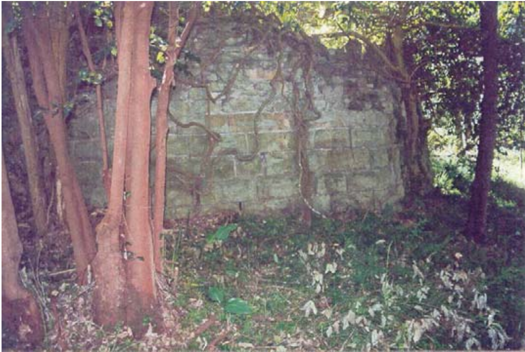
Figure 127: The southern face of the retaining wall supporting the croquet lawn. This section of the retaining wall is much higher than at the northern end of the field, due to the fall in ground level along the base of the wall (Mayne-Wilson & Associates, August 2000).
