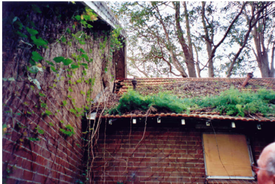
Figure 143: Collapsed section of roof on the south-eastern side of the former Stable (Rod Howard & Associates, 2006).
