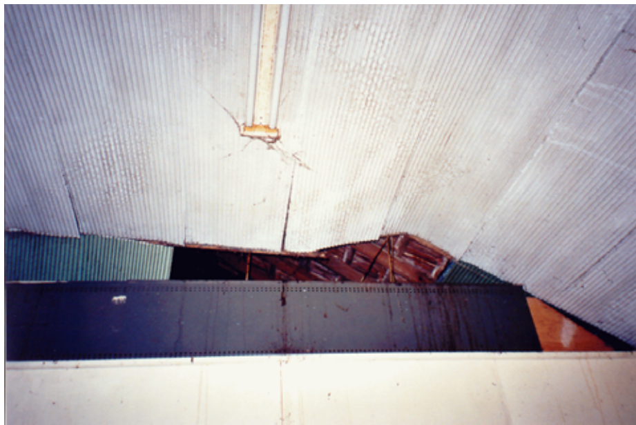
Figure 144: Condition of ceiling linings within the former Stable (Rod Howard & Associates, 2006).
