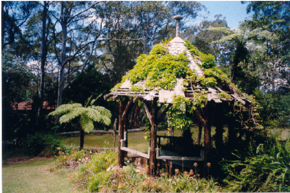
Figure 67: The Summerhouse, on the northern side of the former croquet lawn, was a charming structure that skilfully combined found timber elements with joinery items. It had deteriorated due to a lack of maintenance and the deleterious effects of vegetation that had grown over it (Rod Howard Heritage Conservation Pty Ltd, October 2000).
