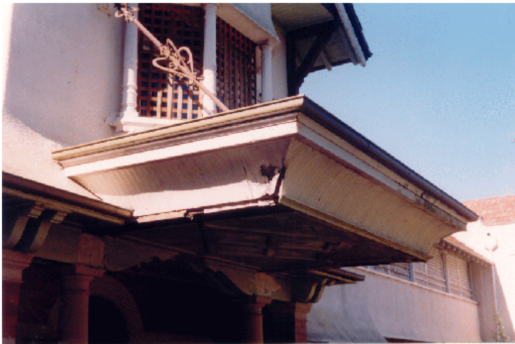
Figure 30: The canopy over the main entrance is deteriorating and has suffered the loss of important elements including the brackets that connect it to the columns on either side of the porch (Rod Howard Heritage Conservation Pty Ltd, October 2000).
