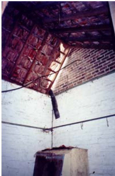
Figure 145: Deterioration of portion of roof within the former Stable (Rod Howard & Associates, 2006).
