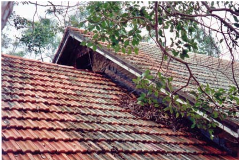
Figure 146: The gap between flashings and lower roof indicate the extent to which the roof has dropped (Rod Howard & Associates, 2006).
