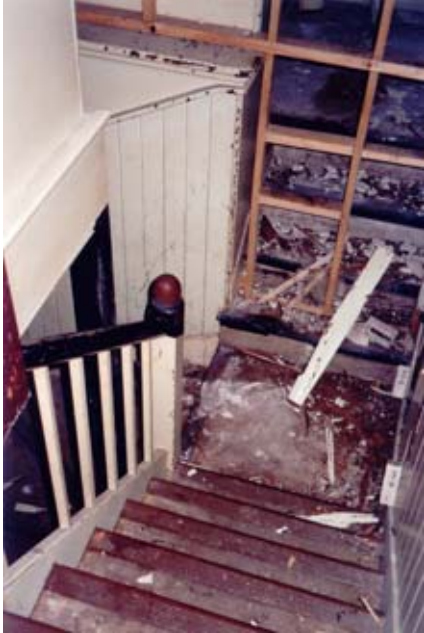
Figure 141: Badly damaged fabric associated with spaces adjacent to the stair at the southern end of “Rippon Grange” (Rod Howard & Associates, 2006).
