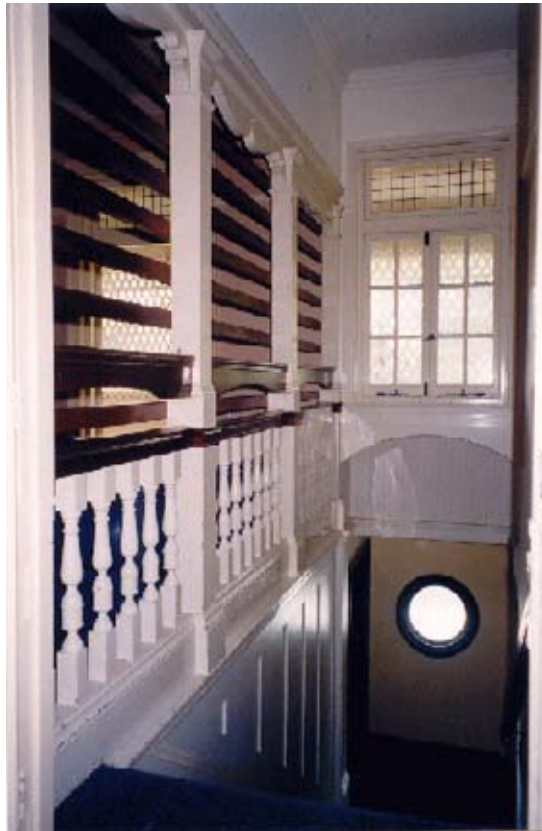
Figure 55: Although much of the joinery relating to the main stair is intact, the spatial quality around Room F18 has been disfigured by the introduction of security screening (Rod Howard Heritage Conservation Pty Ltd, October 2000).
