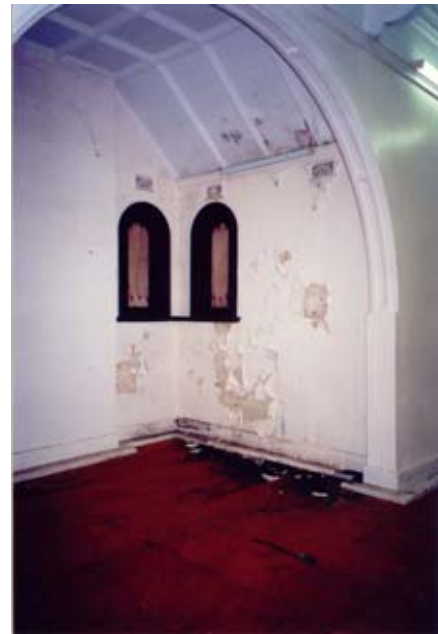
Figure 140: Damaged skirtings and wall surfaces in the north-western corner of Room G4 (Rod Howard & Associates, 2006).
