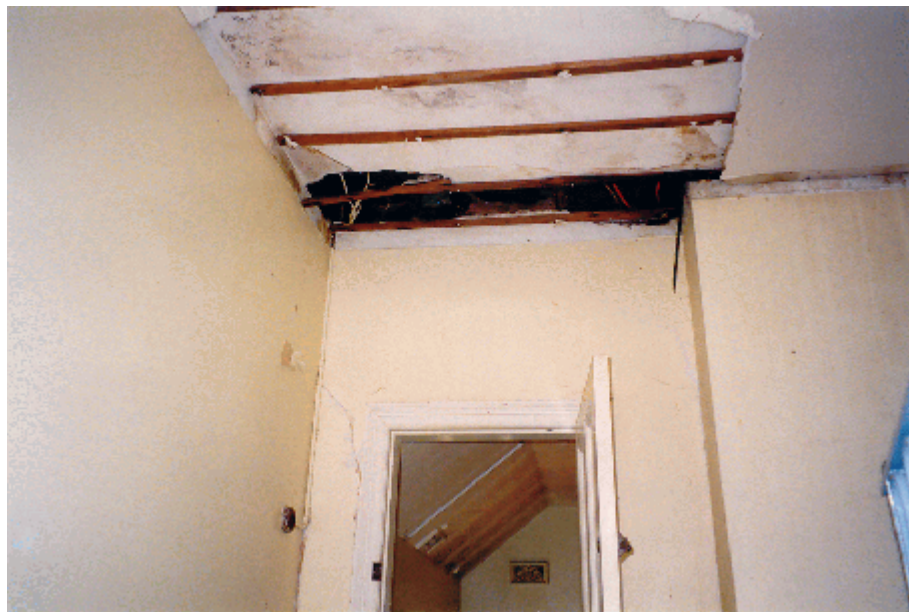
Figure 57: The fabric of Room F19 to F21 has deteriorated as a result of water penetration and other causes. Ceilings have collapsed in some places (Rod Howard Heritage Conservation Pty Ltd, October 2000).
