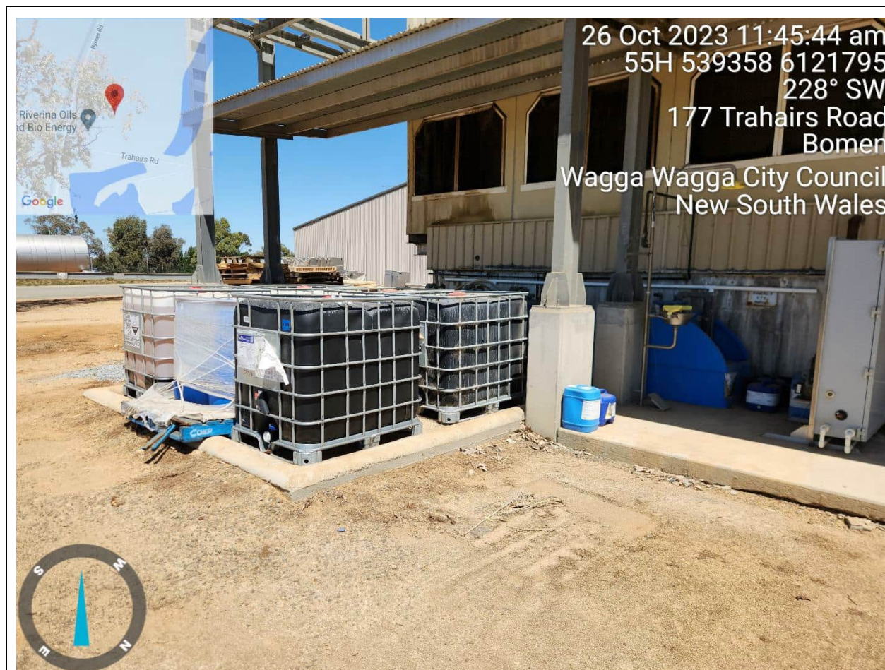
Photo 69: Cooling tower water treatment chemicals
