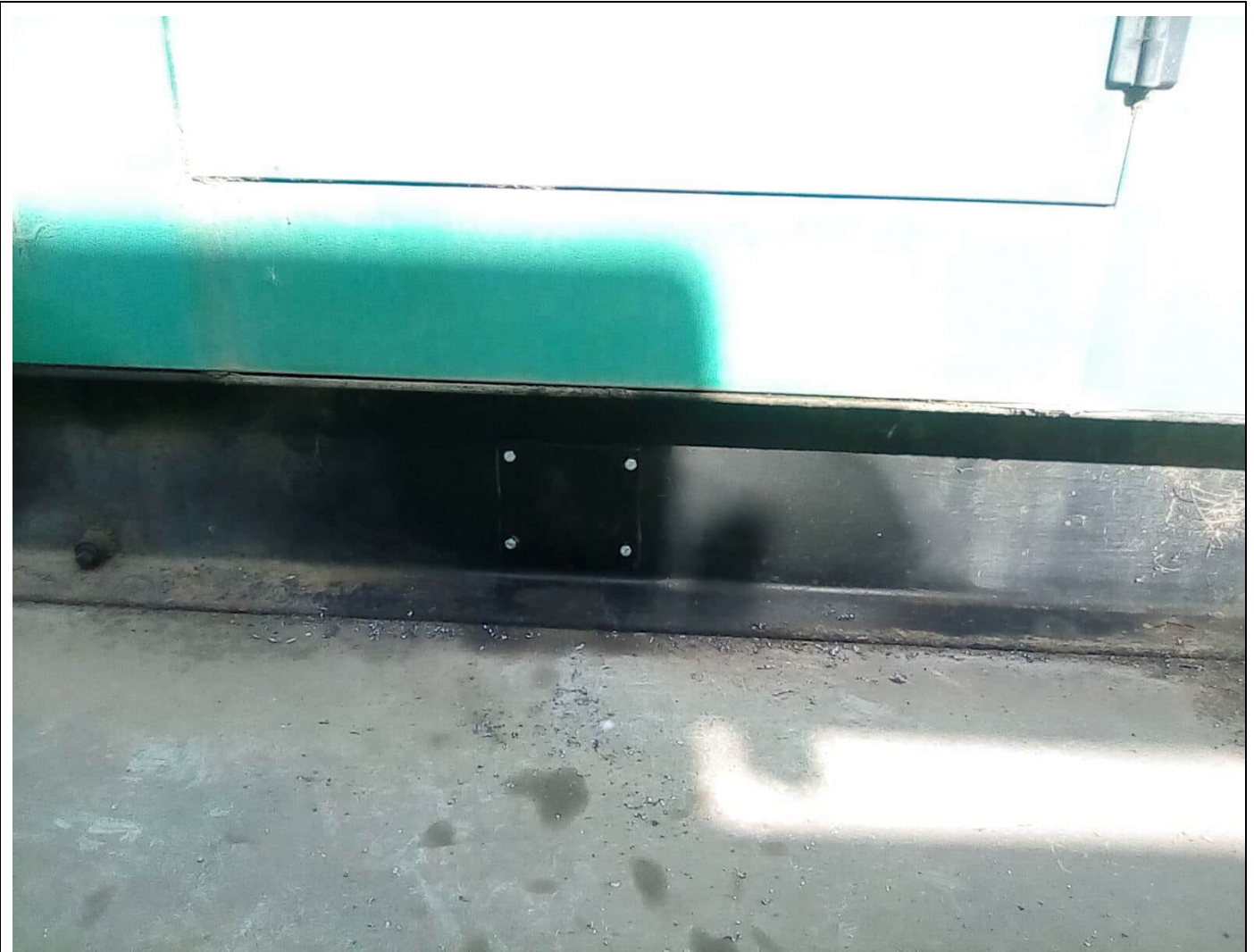
Photo 17: Backup generator 2 bund drainhole
