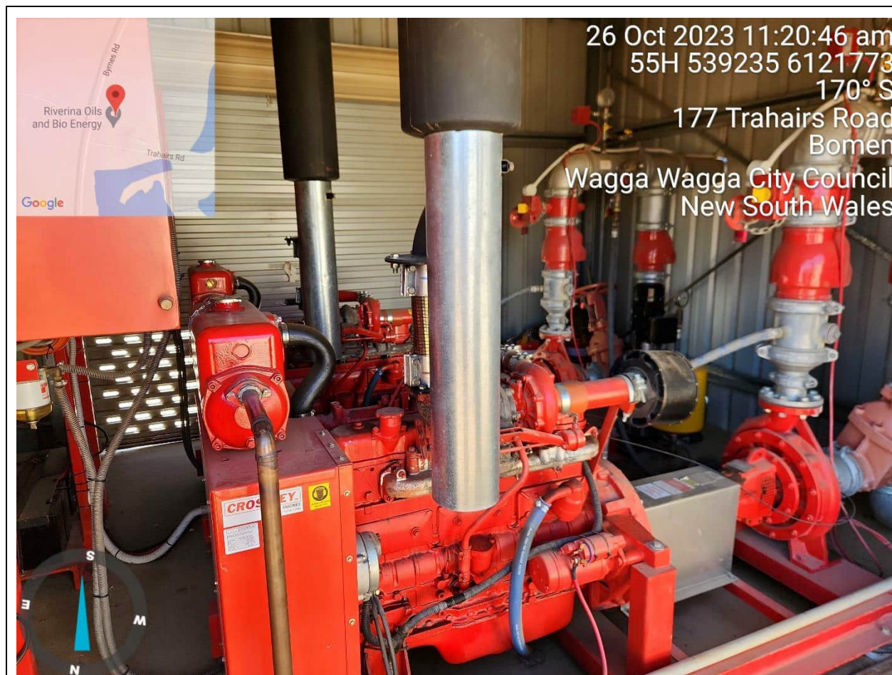
Photo 67: Firefighting water pumps
