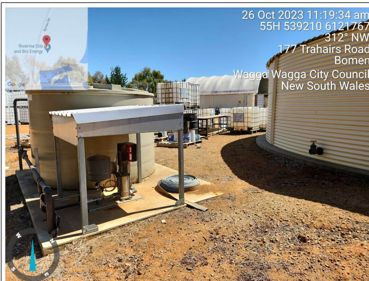
Photo 64: Firefighting water tank
