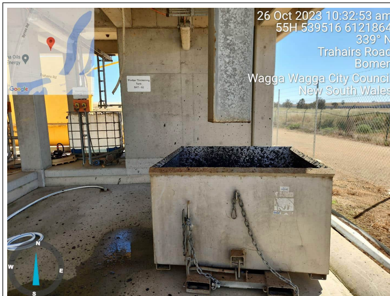
Photo 45: Spent bleaching earth
