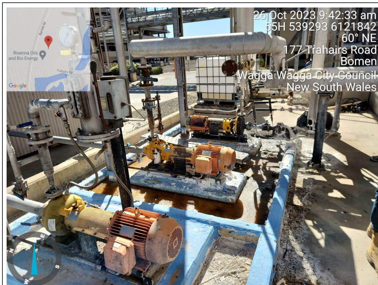
Photo 8: Acid and caustic pumps
