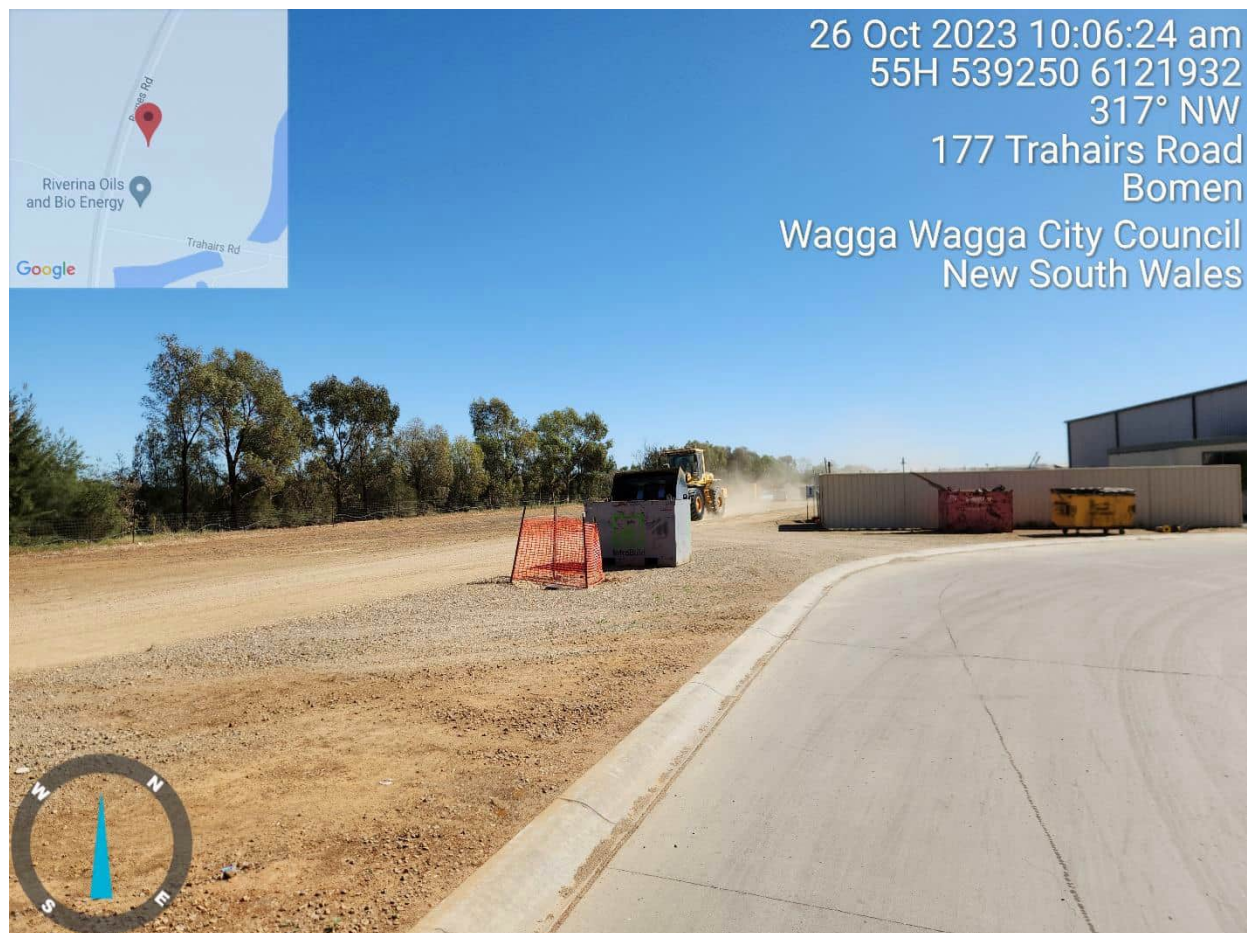
Photo 24: Access track to bulk grain storage - note dust generation
