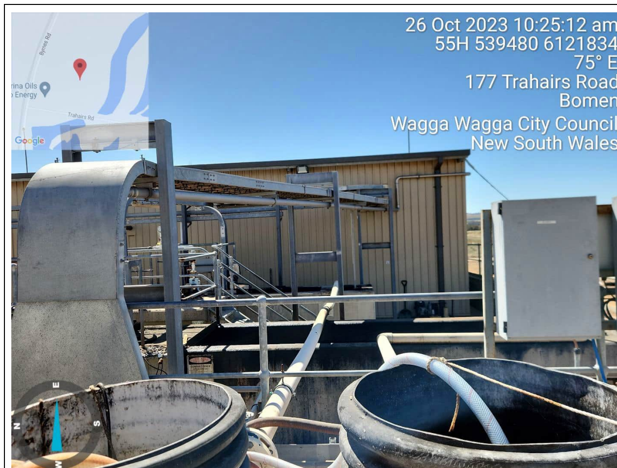
Photo 40: Wastewater treatment plant
