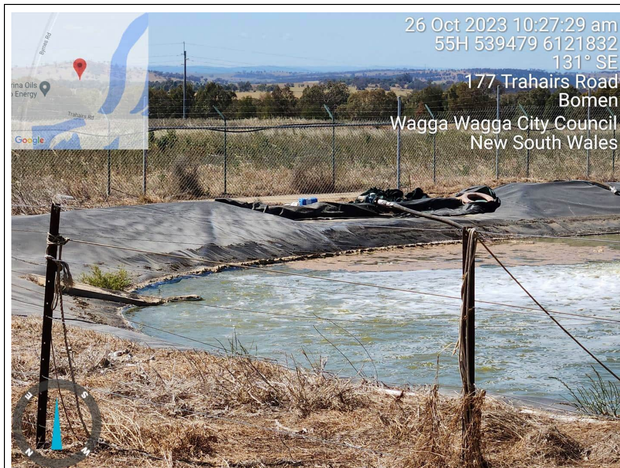
Photo 43: Wastewater storage pond overflow
