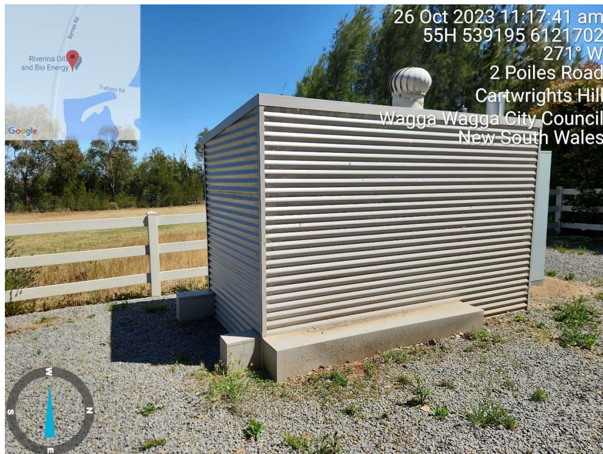
Photo 62: Sewage treatment plant
