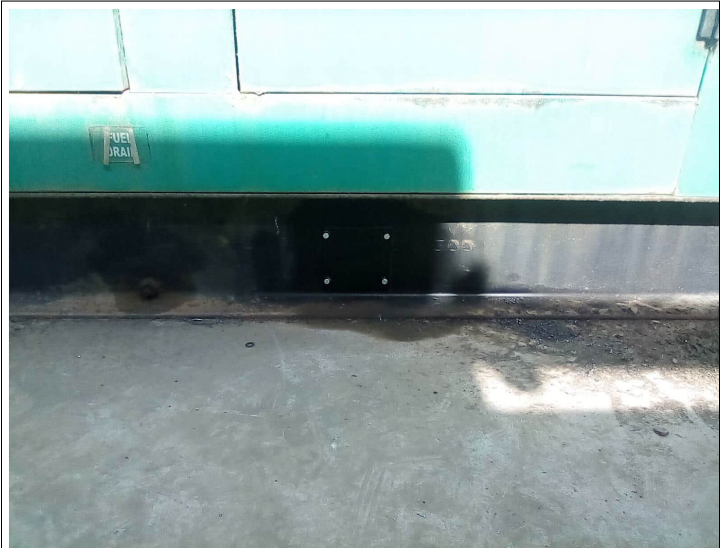
Photo 18: Backup generator 3 bund drainhole
