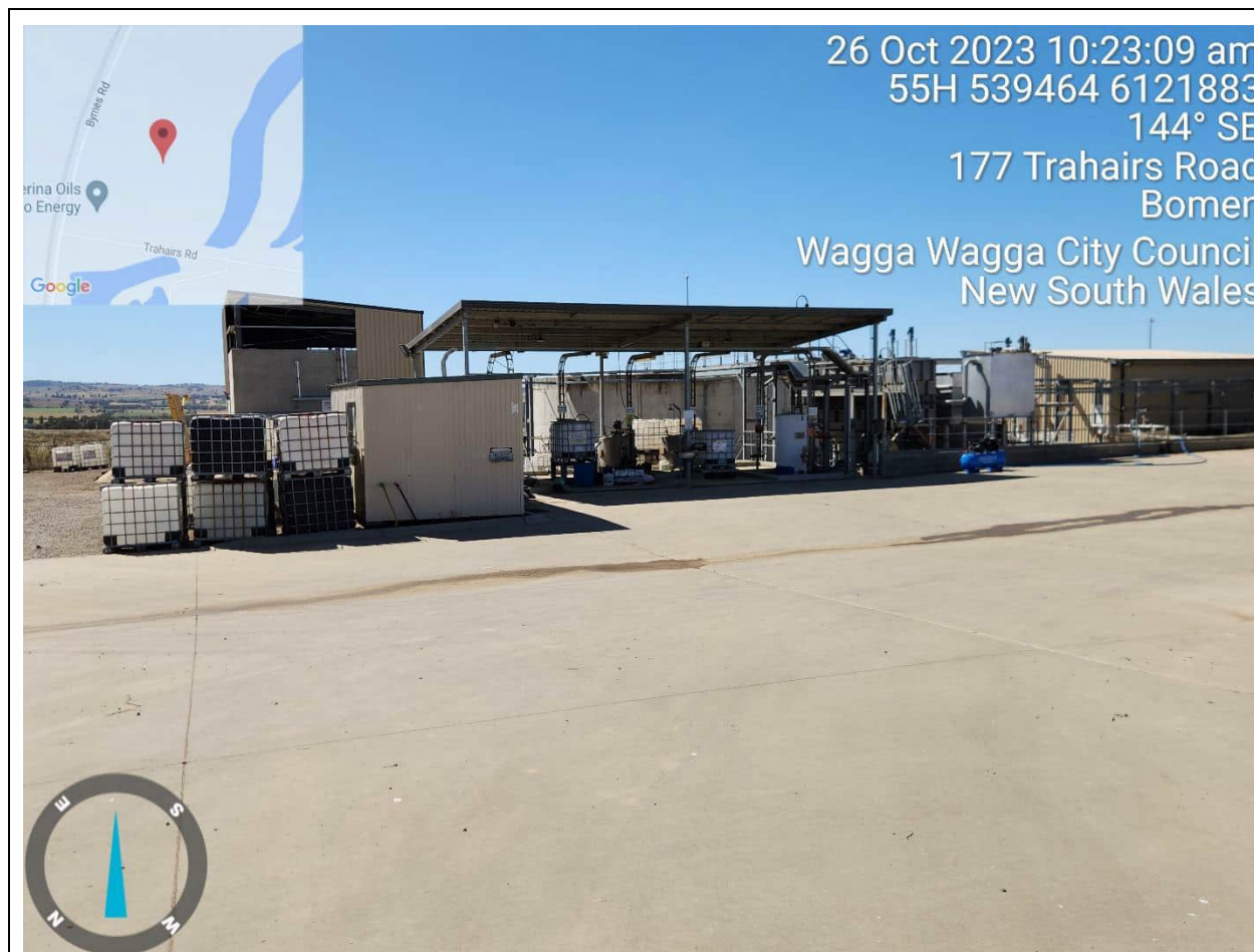
Photo 37: Wastewater treatment plant
