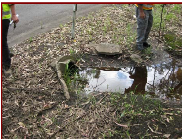
Figure 16. Disturbance from drainage culverts along O'Connell Street, transect 6. .
