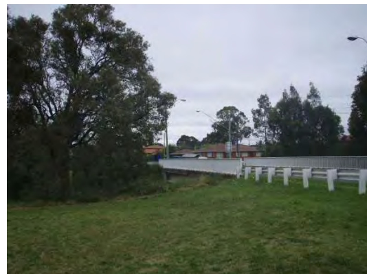
Plate 4: Bridge crossing over Prospect Creek between Normanby Street and Crown Street, Fairfield East. View faces southwest.
