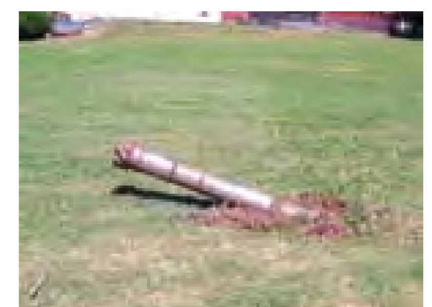
The tip of a horizontal directional drill emerging on the other side of a waterway
