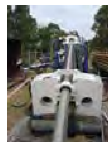
A horizontal directional drill rig being used to drill a hole underneath a major waterway
