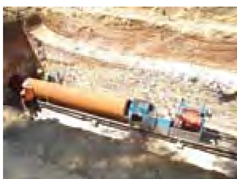
A cased bore being use to install a pipe underneath a major roadway to minimise traffic disruptions
