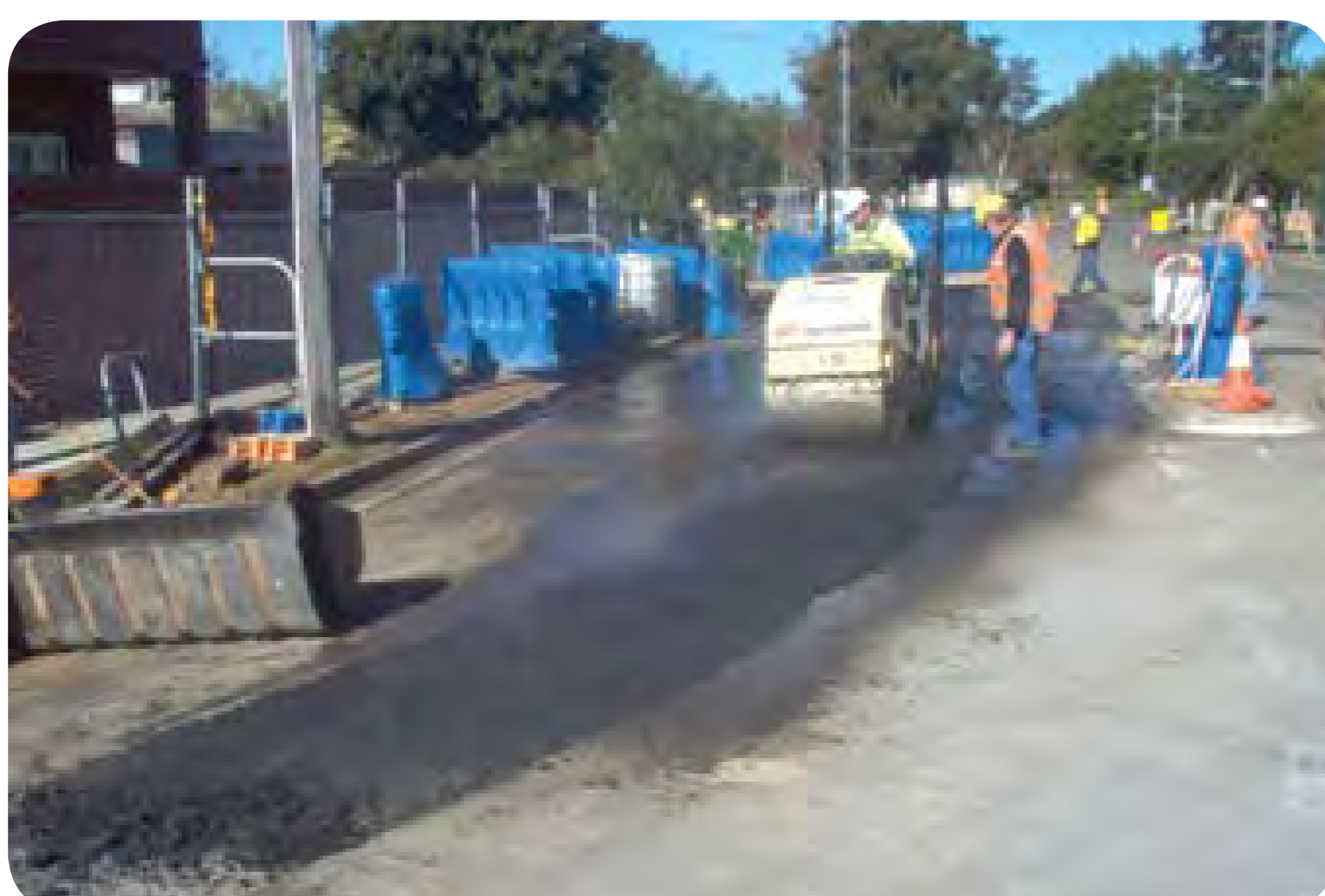
A temporary restoration being carried out for a trench in a roadway
