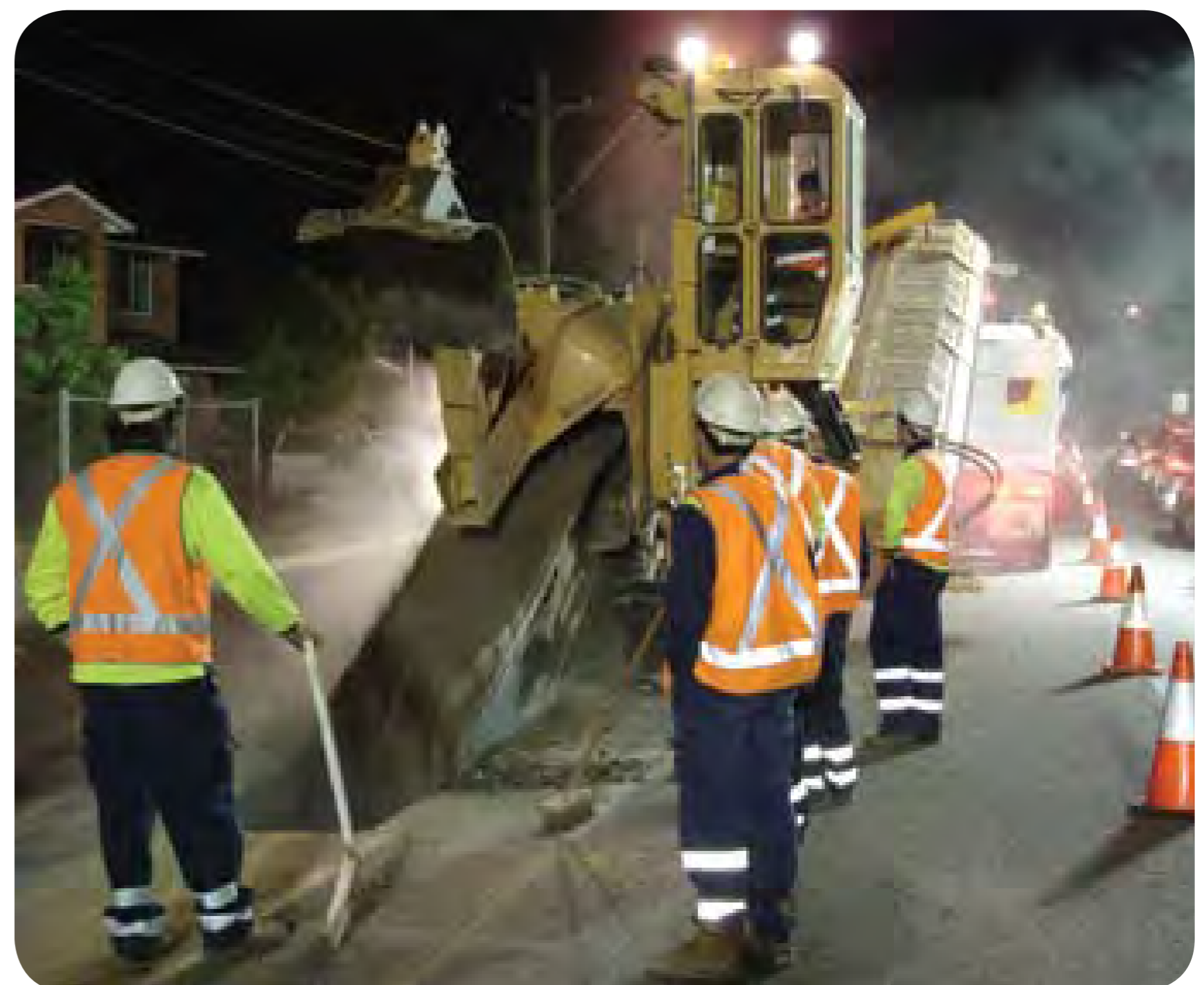
Along busy roads, trenching work may occur at night to minimise disruptions to traffic
