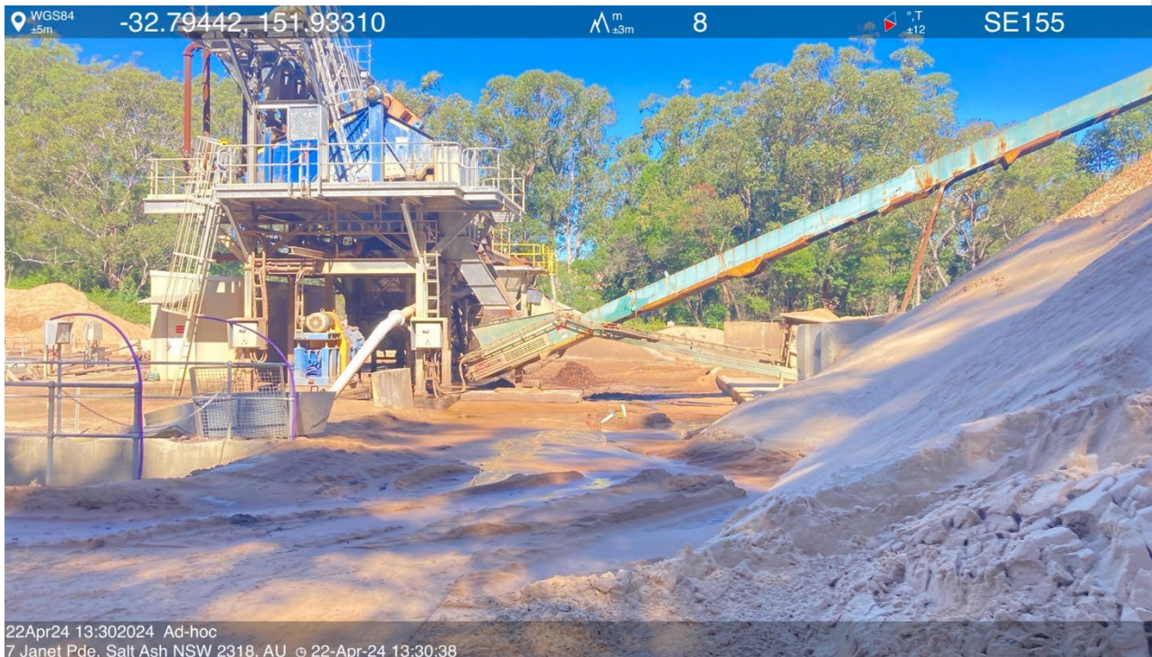
Sand screening and wash plant
