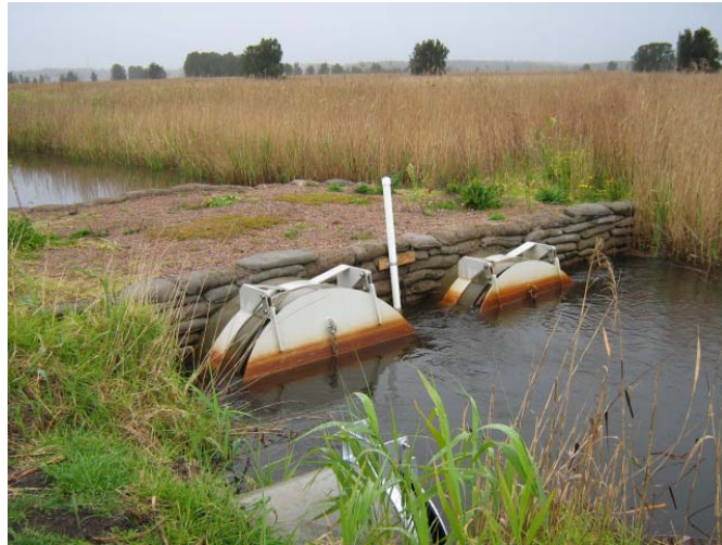
Plate 3 – Twin 1500mm pipe crossing
