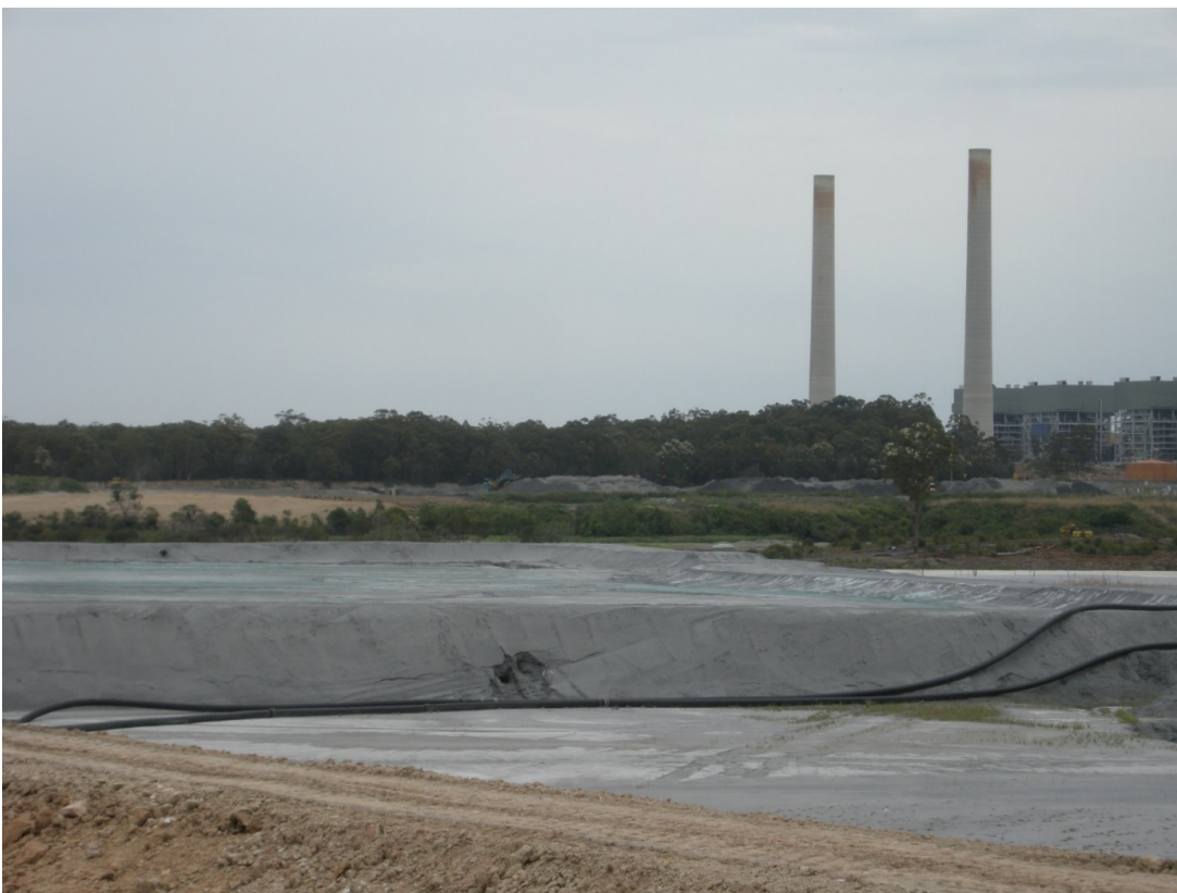
Figure 3.4 "Piping" in ash cell wall
