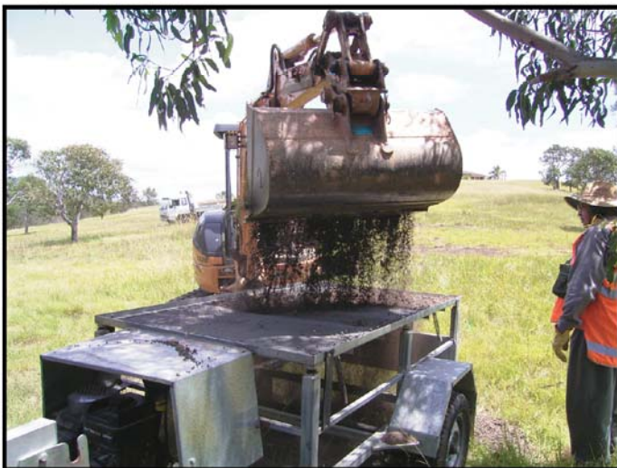
Plate 5. Excavated sediments placed directly on mechanically-agitated sieve (TP A/4 in central section of the investigation area).
