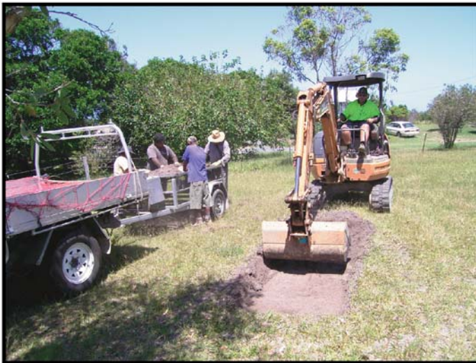
Plate 3. Typical excavation procedure (TP B/6 on southern end of the investigation area).
