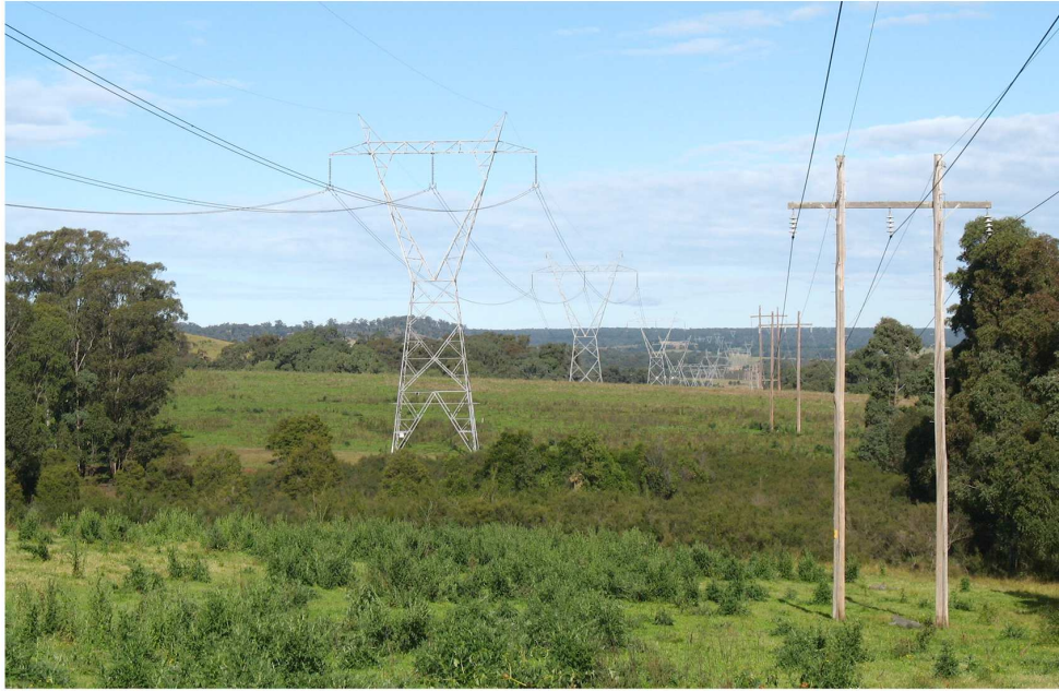
Photograph taken from Leafs Gully Road looking South: 330kV and 66kV powerlines. The 330kV powerline towers (on the left hand side of photo) are approximately 45 metres high
