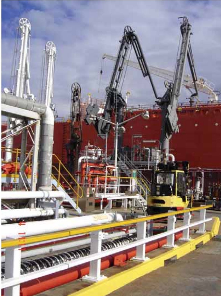
■ Figure 4-5 Existing MLAs at BLB1
