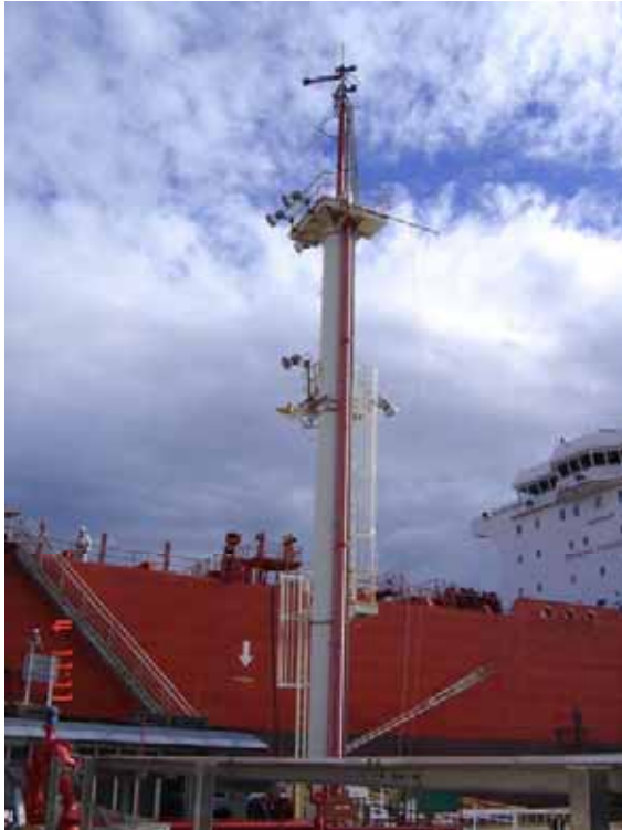
■ Figure 4-6 Existing Fire Monitor at BLB1
