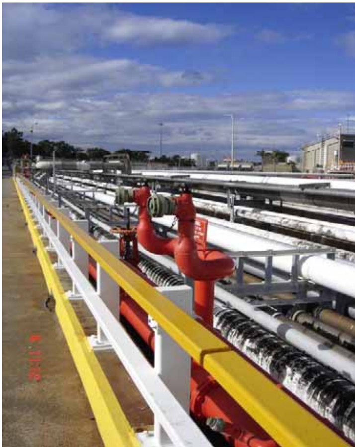
■ Figure 4-7 Existing Pipelines at BLB1
