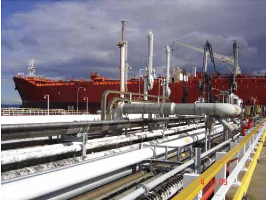
Figure 1-1 View of equipment infrastructure at BLB1
