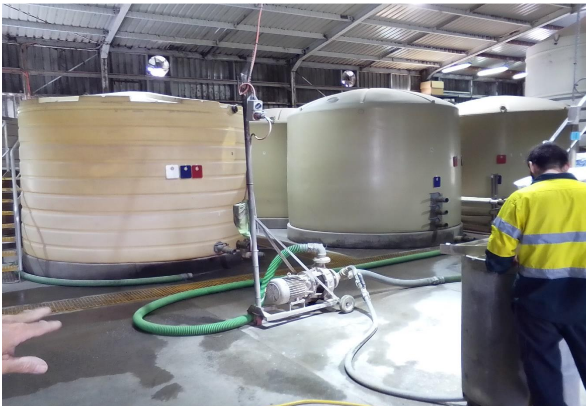
Plate 12 Grease trap waste storage tanks inside Treatment Shed
