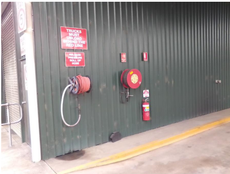
Plate 4 Fire fighting equipment available and in good condition within Truck Receival area
