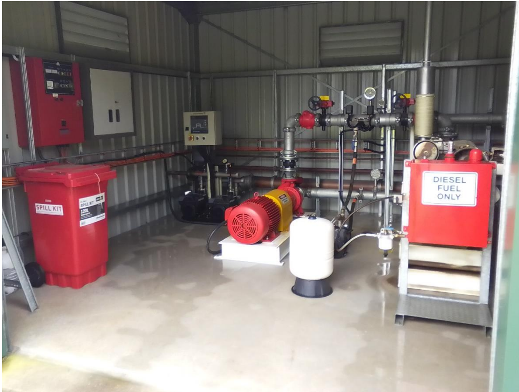
Plate 5 Fire fighting system in place and in good condition
