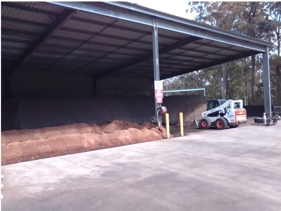
Plate 6 Waste Storage Drying Bay
