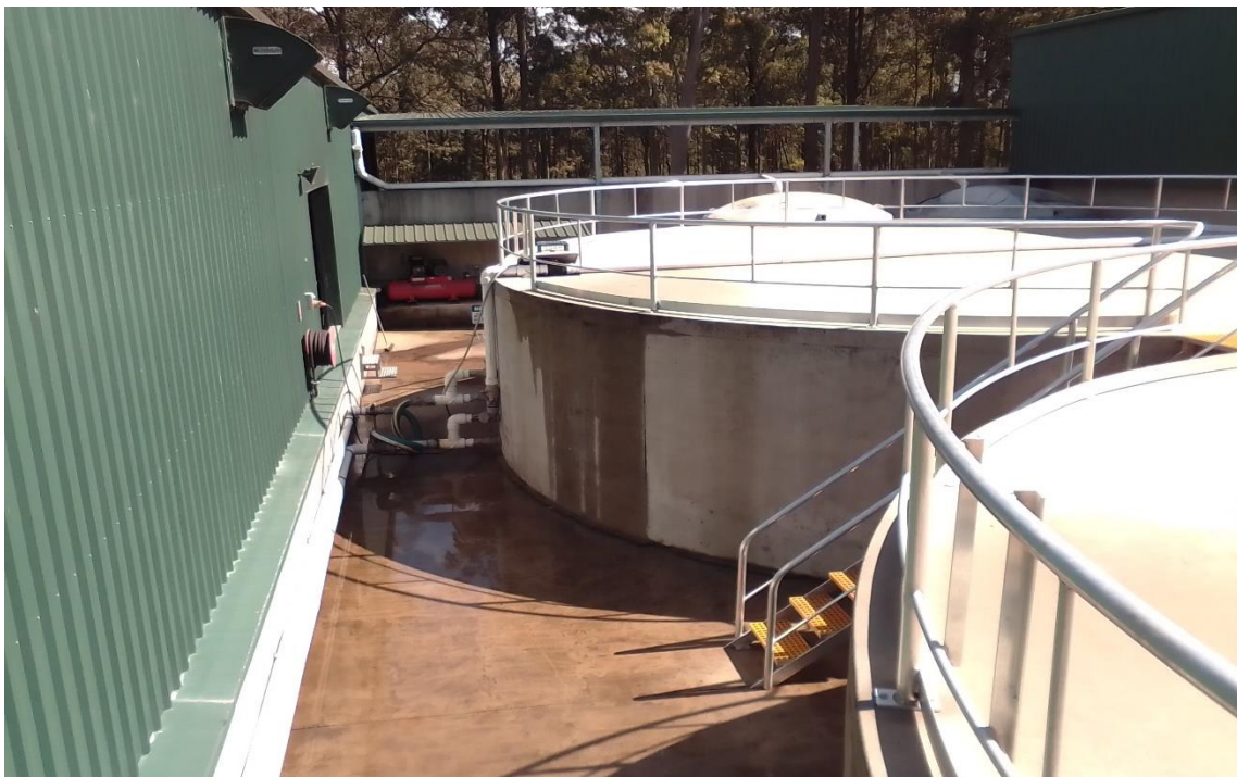
Plate 10 Rainwater / Contingency Storage Tanks
