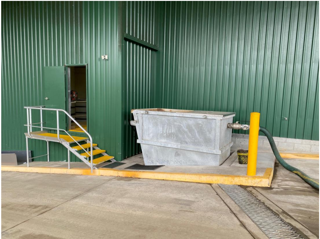
Figure 5 Screening and sediment bin on the eastern side of the building.
