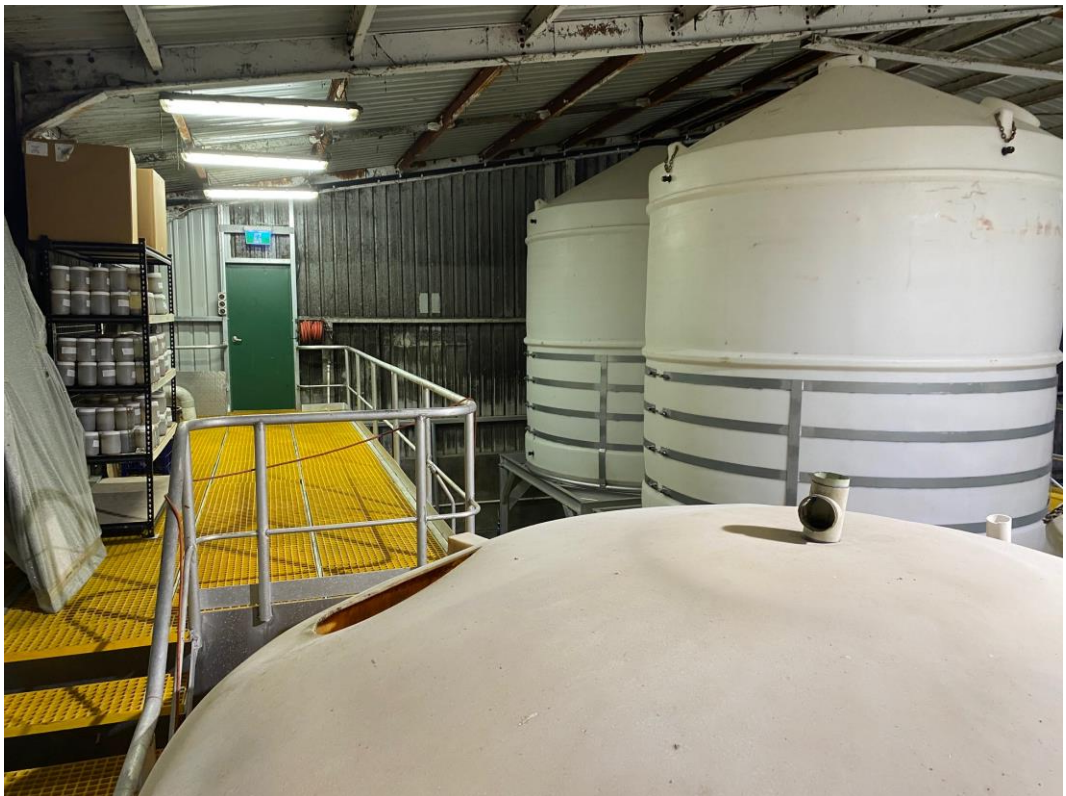
Figure 6 Receiving Tanks 2 and 3.
