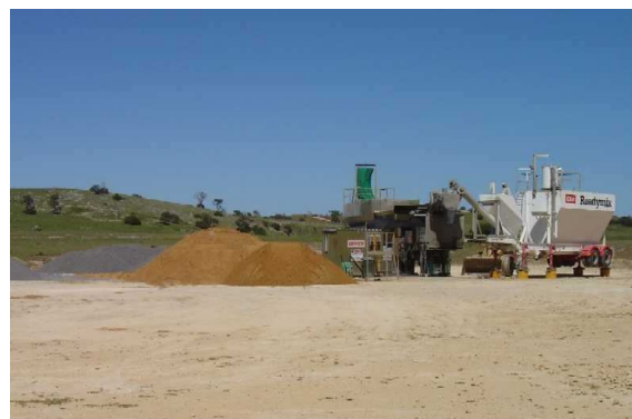
Plate 3.4 Typical Portable Concrete Batch Plant
