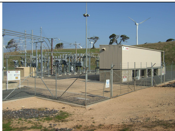
Plate 3.2 Typical substation building housing switchgear within secure compound
