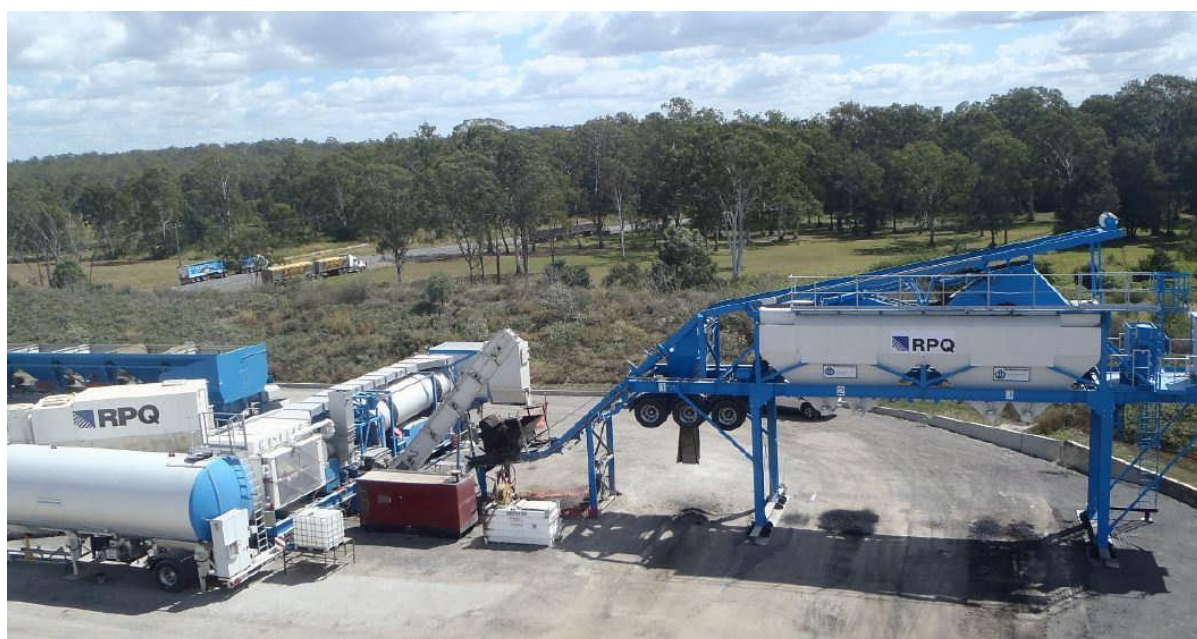
Figure 3 | Asphalt plant equipment
