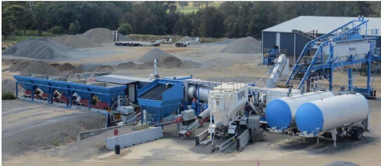
Figure 4 | Asphalt plant equipment
