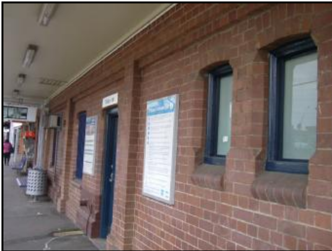
Photograph 8: Southern elevation of Beverly Hills Railway Station showing bullnose window sills and design features
