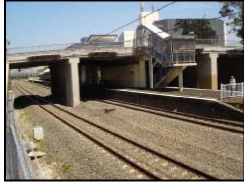
Figure 6 Kingsgrove station with its 4-span overbridge, the inner two spans are jack arch, side span are concrete.
