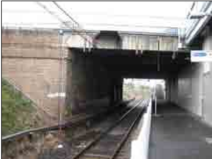
Photograph 12: King Georges Road overbridge brick abutment and central pier on the island platform
