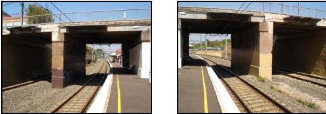
Figures 8 and 9 At Bardwell Park station the whole platform follows the left-hand curve of the railway corridor. The platform edges are parallel left-hand curves, not opposite hand as with a symmetrical platform. The Bardwell Park platform is non-symmetrical.
